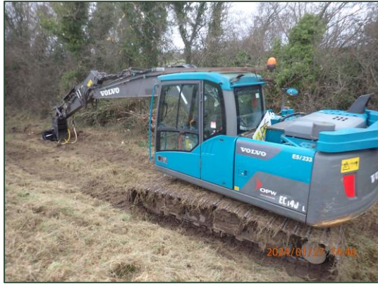
Plate 3.7 Excavator undertaking riparian vegetation clearance in close proximity to Otter holt along the Greanagh River.
