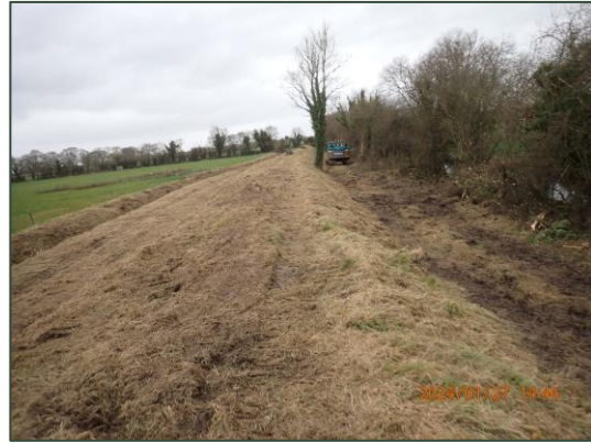
Plate 3.8 View of excavator clearing vegetation along the Greanagh River in proximity to known Otter holt.
