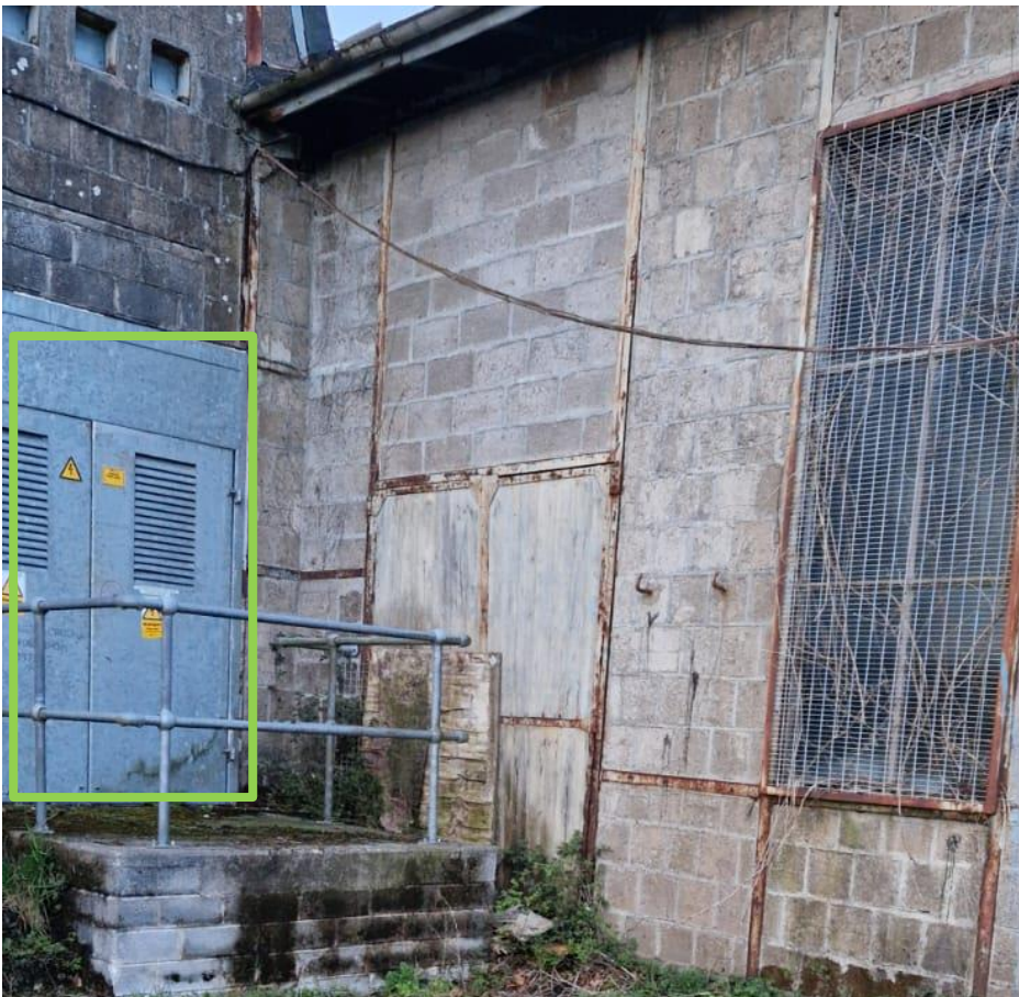
Plate 1: The steel door entrance to Substation Room (Part C – marked by Green box).
