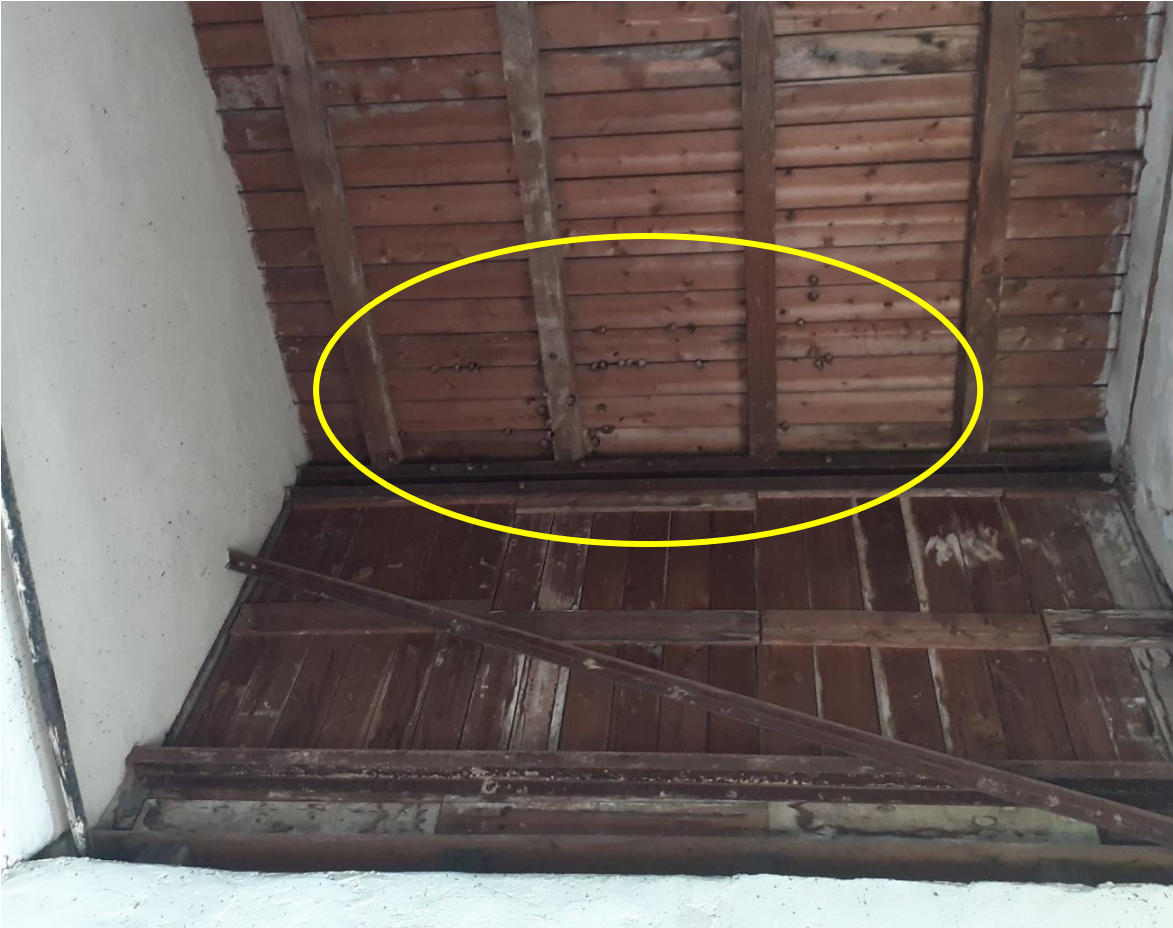
Plate 2: Rafter space in Part C, Substation Room (Lesser horseshoe bats visible – highlighted in yellow). Please note that how high the ceiling space is above the wall plate (i.e. the top of the white painted wall).
