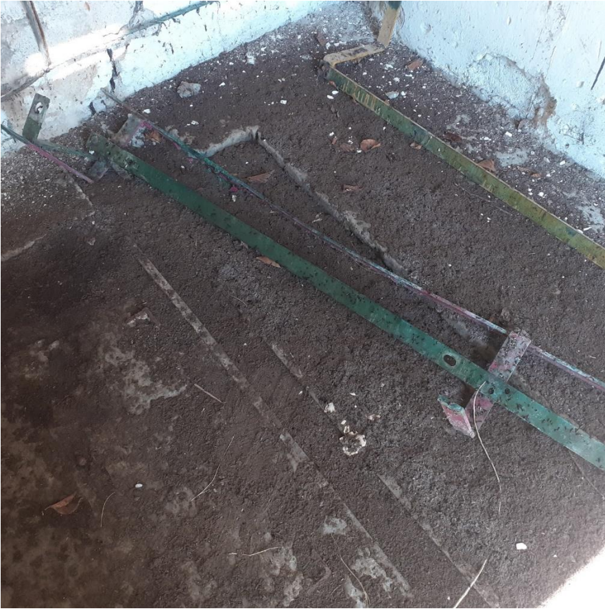
Plate 4: Extent of old bat droppings present on the substation floor (Part C).
