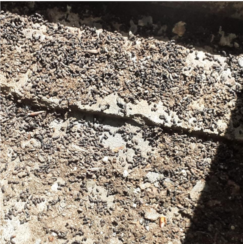
Plate 3: Bat droppings on substation floor (Part D).
