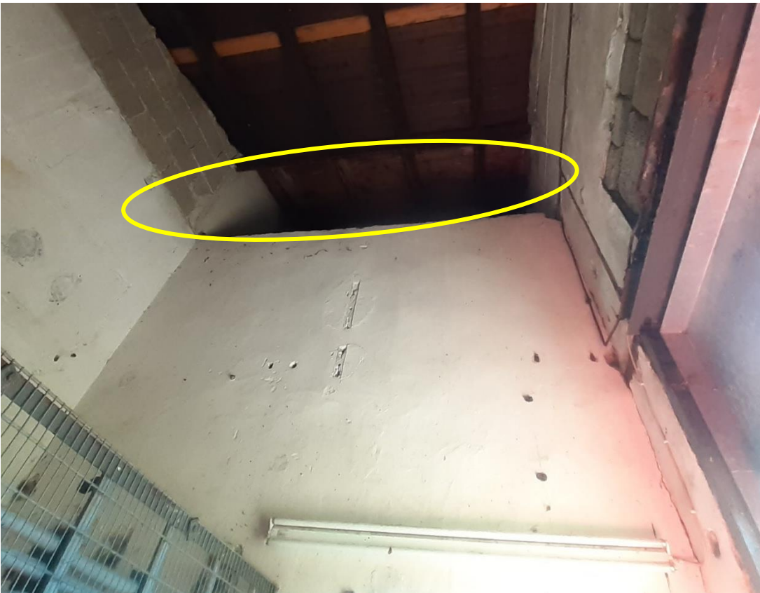
Plate 5: Internal wall in between the two rooms (Part C and Part D) of Substation Room. (Yellow Circle). Please note that how high the ceiling space and the internal white wall (wall between Part C and Part D of the Substation). The steel structure in the right-hand corner is 1.8m high and protects the active equipment of the substation.
