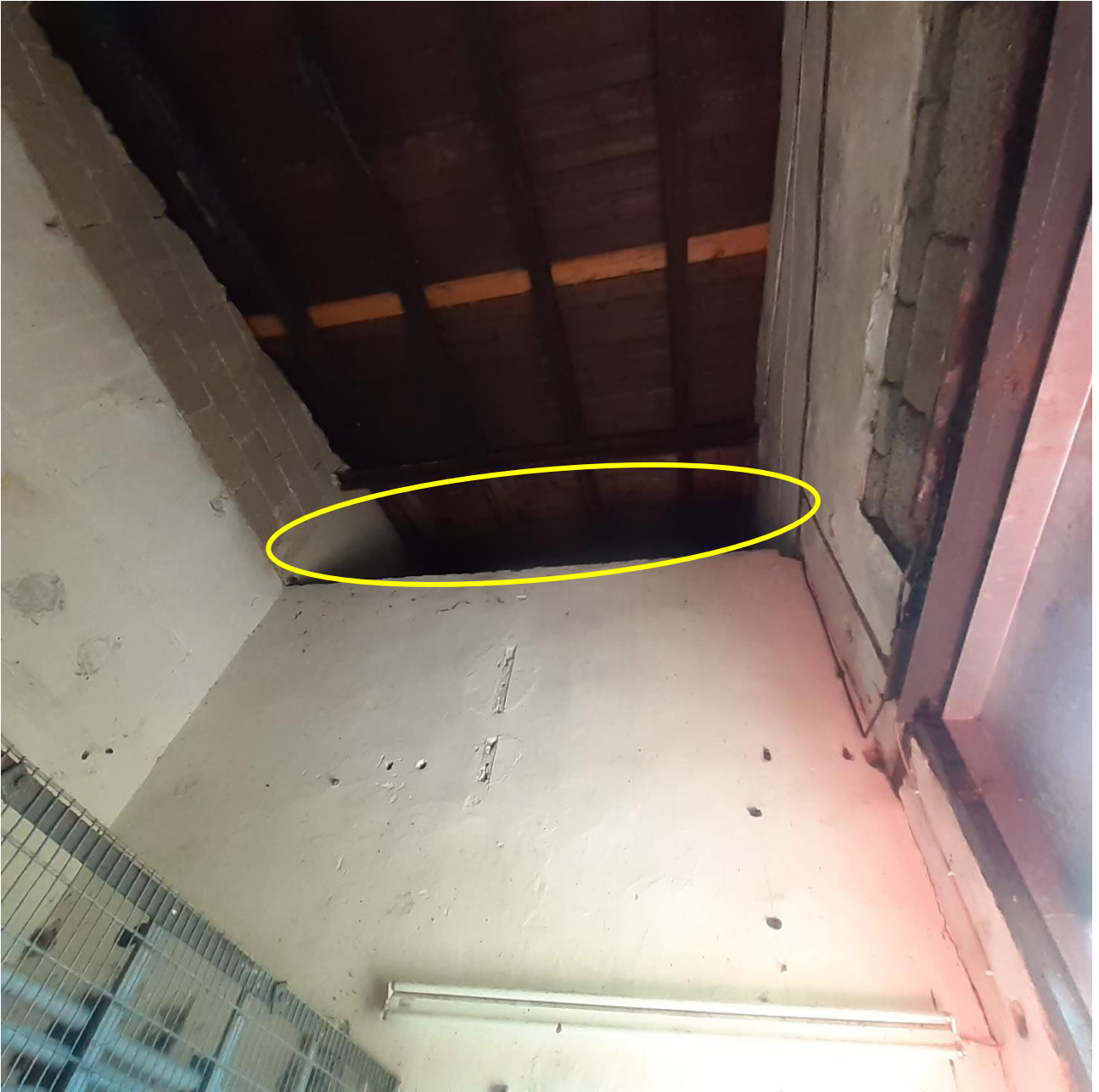
Plate 8: Internal wall in between the two rooms (Part C and Part D) of Substation Room. (Yellow Circle).
