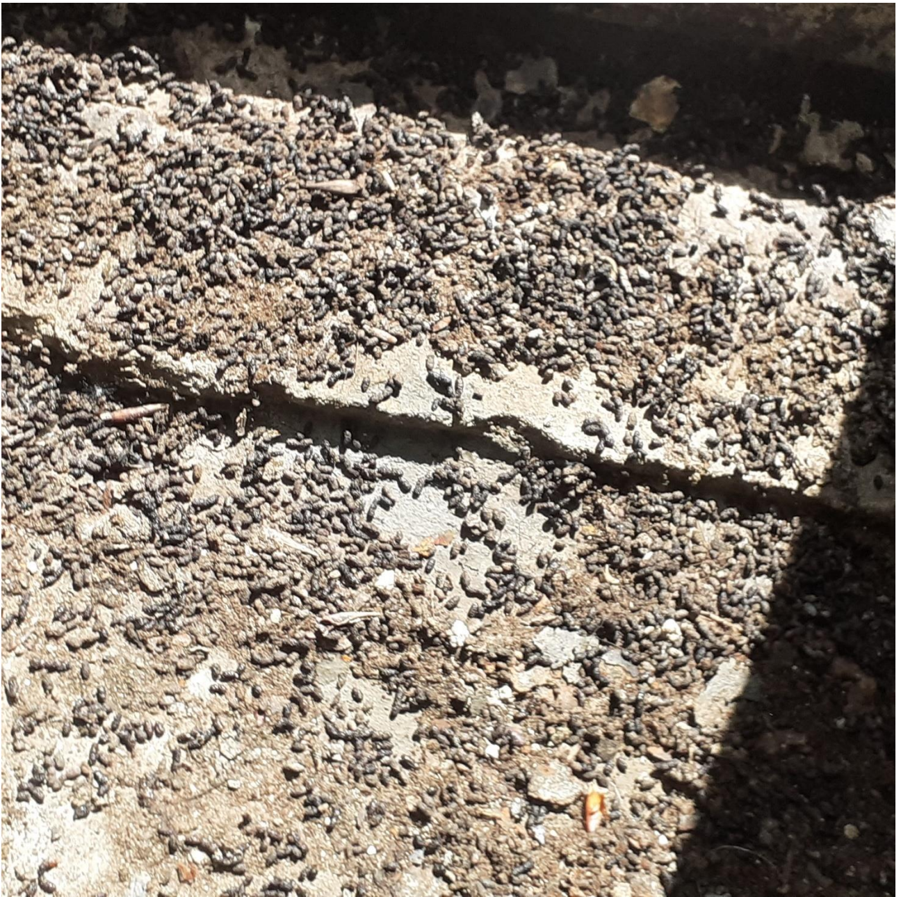
Plate 6: Bat droppings on substation floor (Part D).
