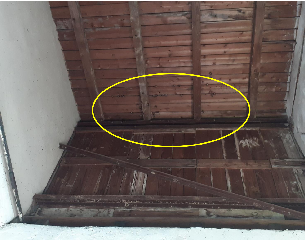
Plate 5: Rafter space in Part C, Substation Room (Lesser horseshoe bats visible – highlighted in yellow).
