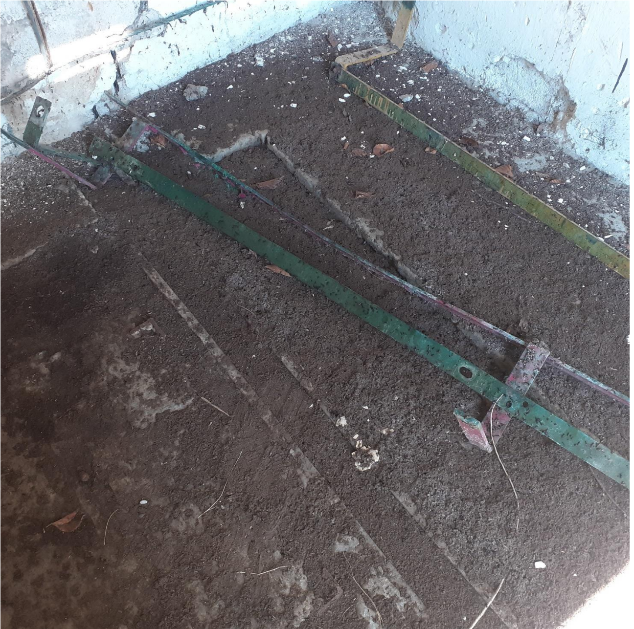
Plate 7: Extent of old bat droppings present on the substation floor (Part C).
