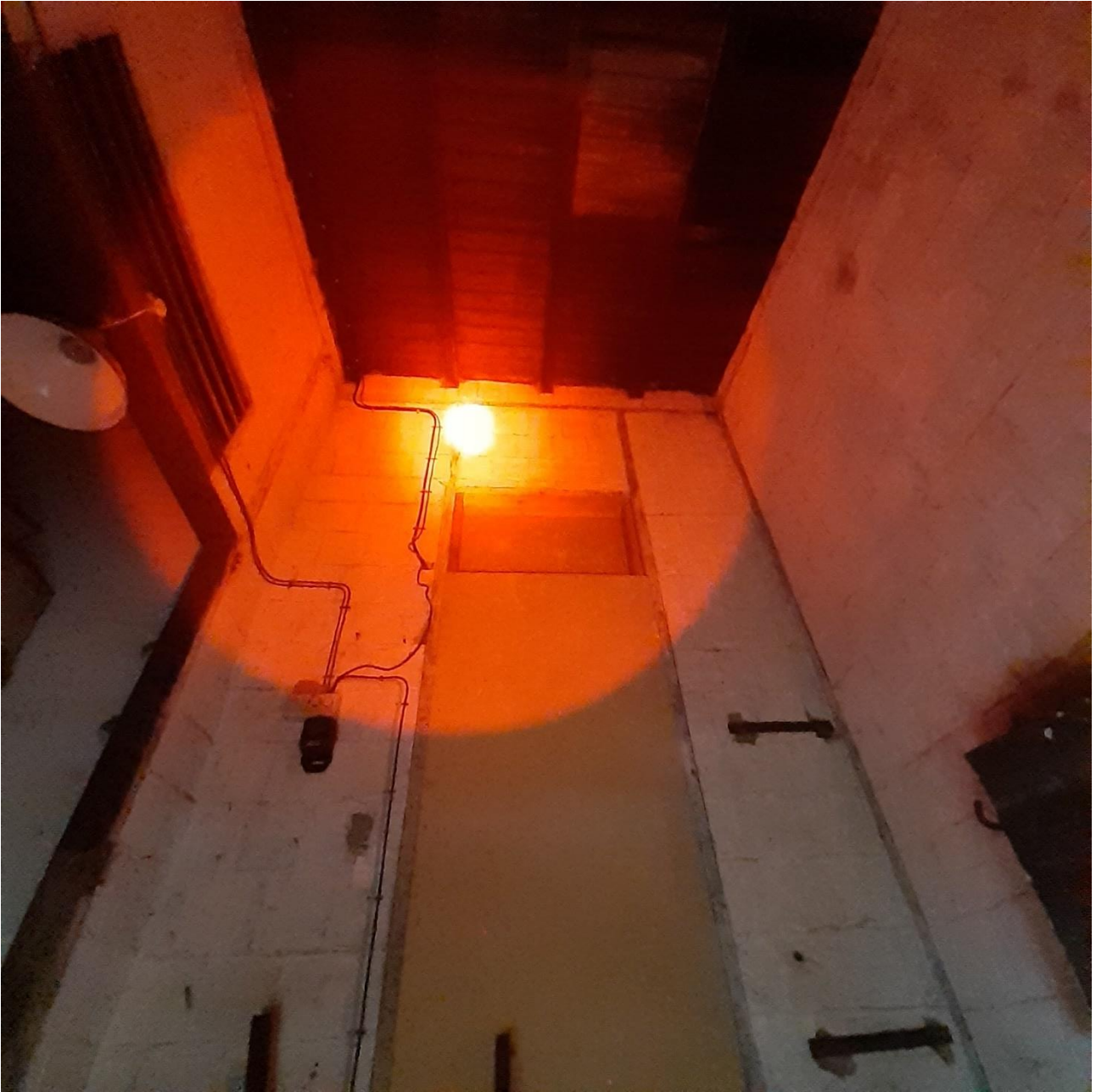
Plate 11: Internal space of Part A, Transition Room (depicting the wall shared with the main space of the Transformer Building. Entrance/Exit into the main space of the Transformer Building is at the rafter level highlighted by the Red Torch.
