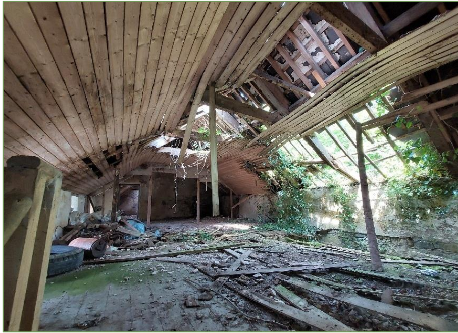
Plate 3.2 Interior view of the two-storey outbuilding (Roost ID: 44) which shows advanced state of dereliction allowing significant light and water ingress into the main roosting location of Lesser Horseshoe Bat.
