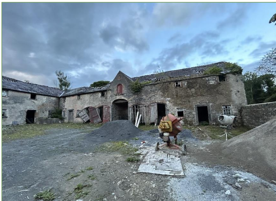
Plate 3.3 View looking east showing the associated stonework structures attached to the two-storey outbuilding containing the Lesser Horseshoe Bat maternity roost (Roost ID: 44).
