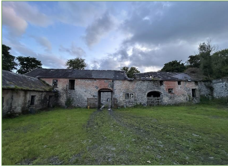
A1. View looking west of the former stables complex and courtyard attached to the Lesser Horseshoe Bat maternity roost (Roost ID: 44).
