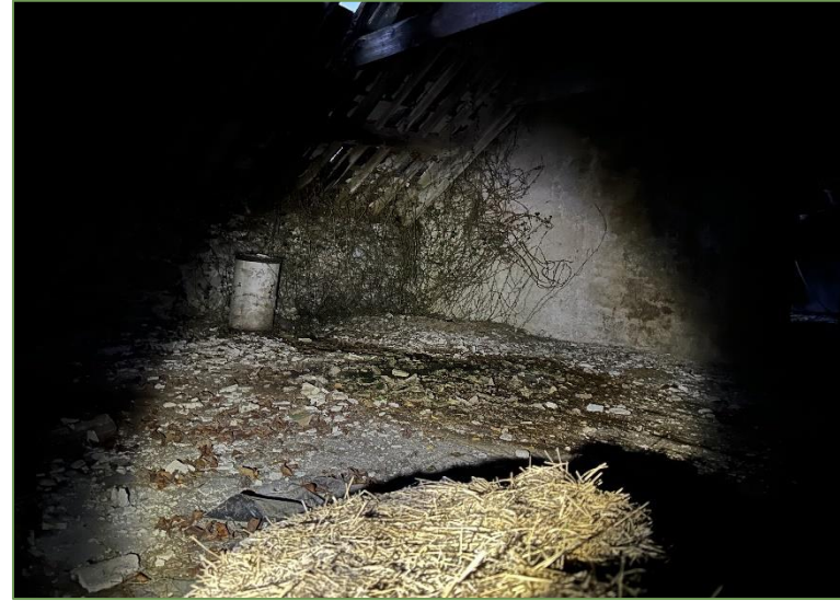
A4. View within the current roosting location for the Lesser Horseshoe Bat maternity colony within Roost ID: 44. Accumulation of droppings and light ingress are clearly visible.
