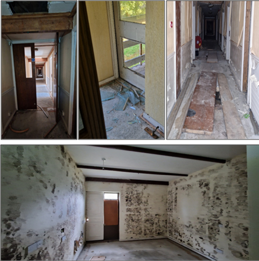
Plate 1 The interior of the two-storey section of the hotel with damage and prevailing damp conditions.
