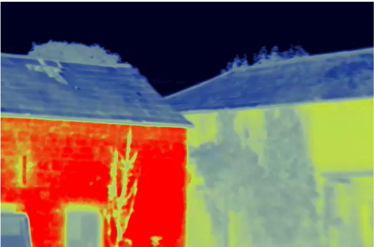
Plate 10: Additional thermal imagery filming of the rear section of stable courtyard building to determine if bats were exiting from the gaps in the slates of the roof – building to right hand-side of screen shot.
