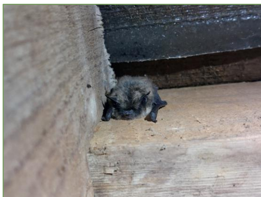
Plate 3.2.9 Whiskered Bat roosting along the ridge beam within the attic of Lissardagh House.
