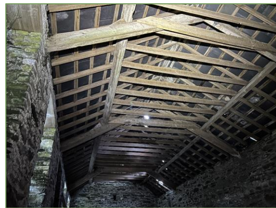
Plate 3.2.4 View of the interior roof space of the Coach House. Note the lack of tile underlay and light ingress.
