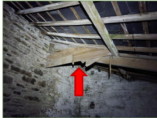
Plate 3.2.6 View of structural timber within outbuilding, of which Brown Long-eared Bat droppings were observed underneath.
