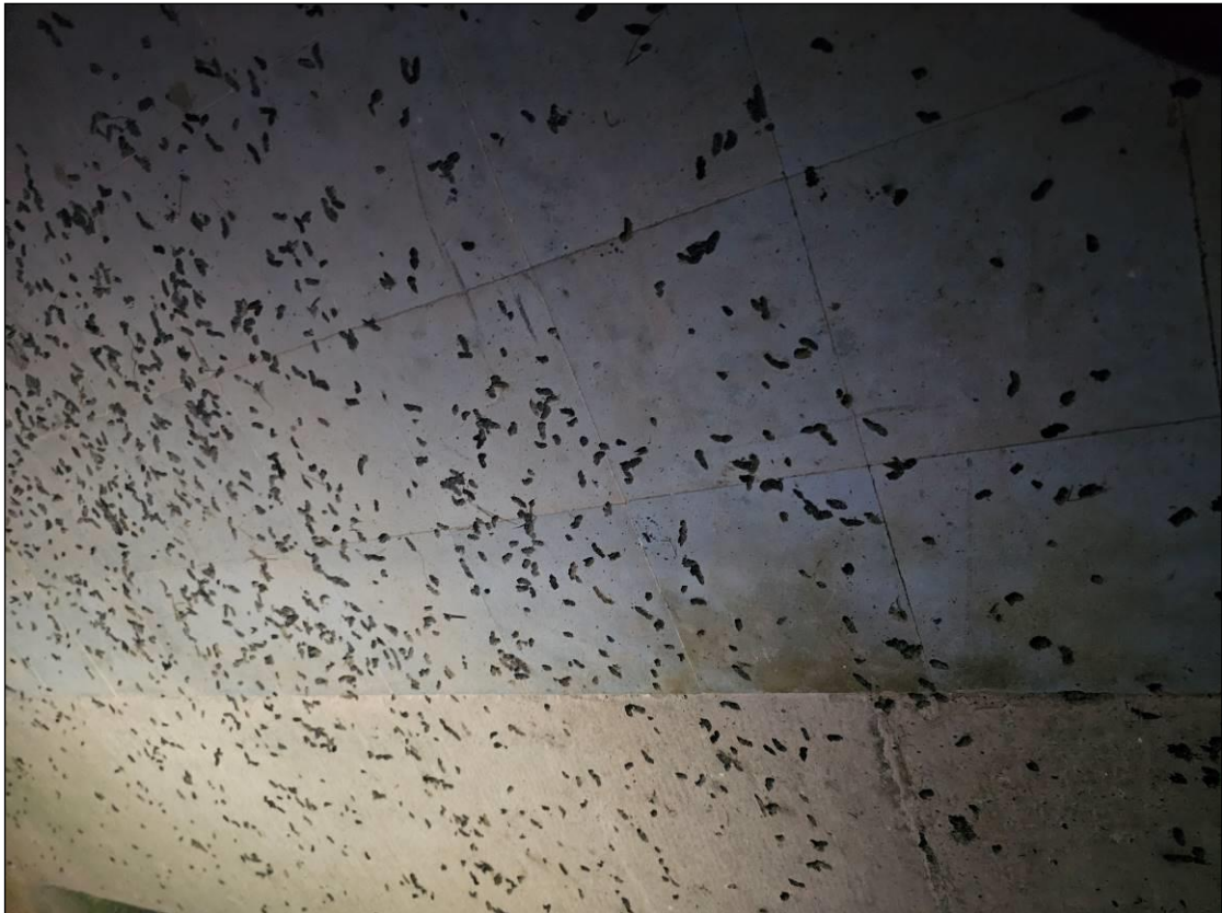
Plate 27. Bat droppings scattered on the floor.
