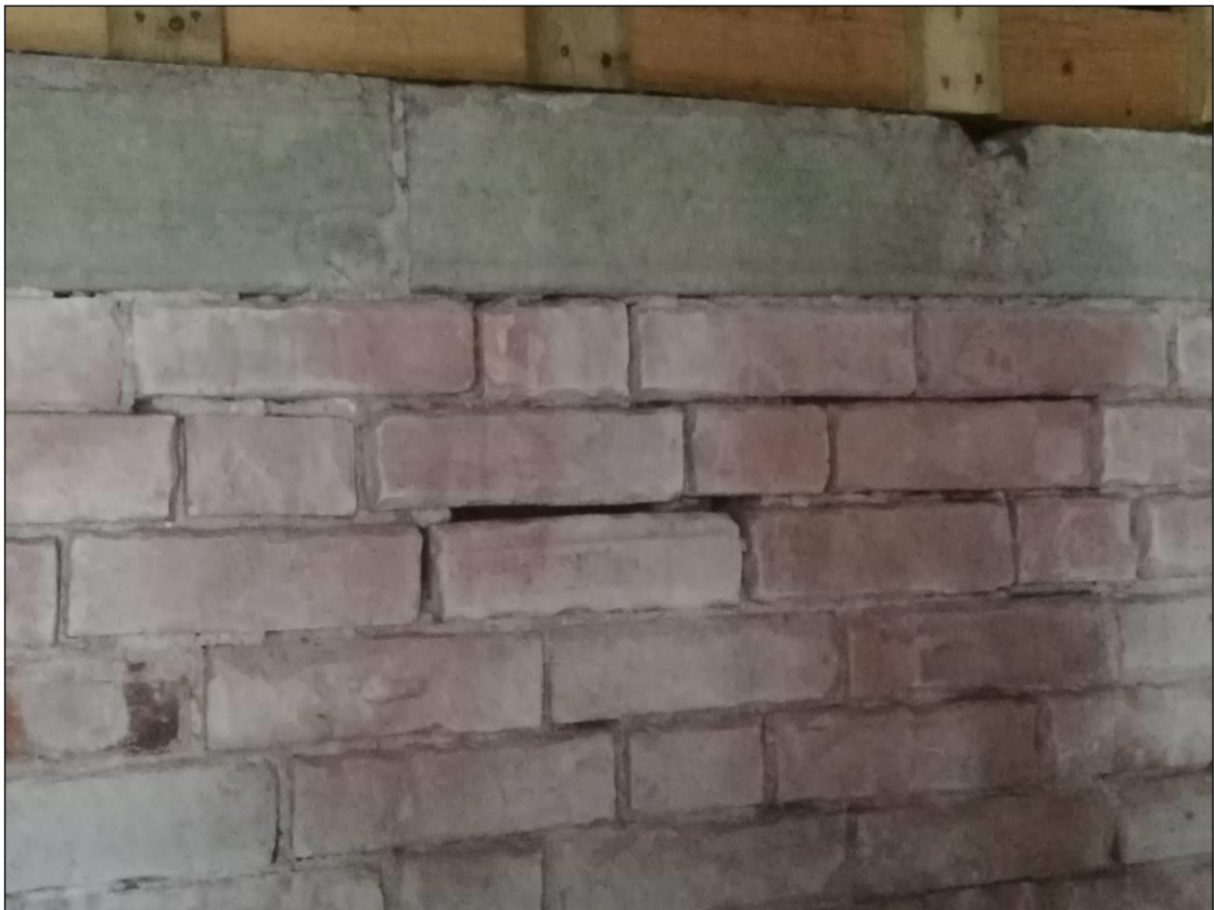
Plate 7. Suitable roosting crevices in brickwork in the side aisles for crevice dwelling bats which should be retained.
