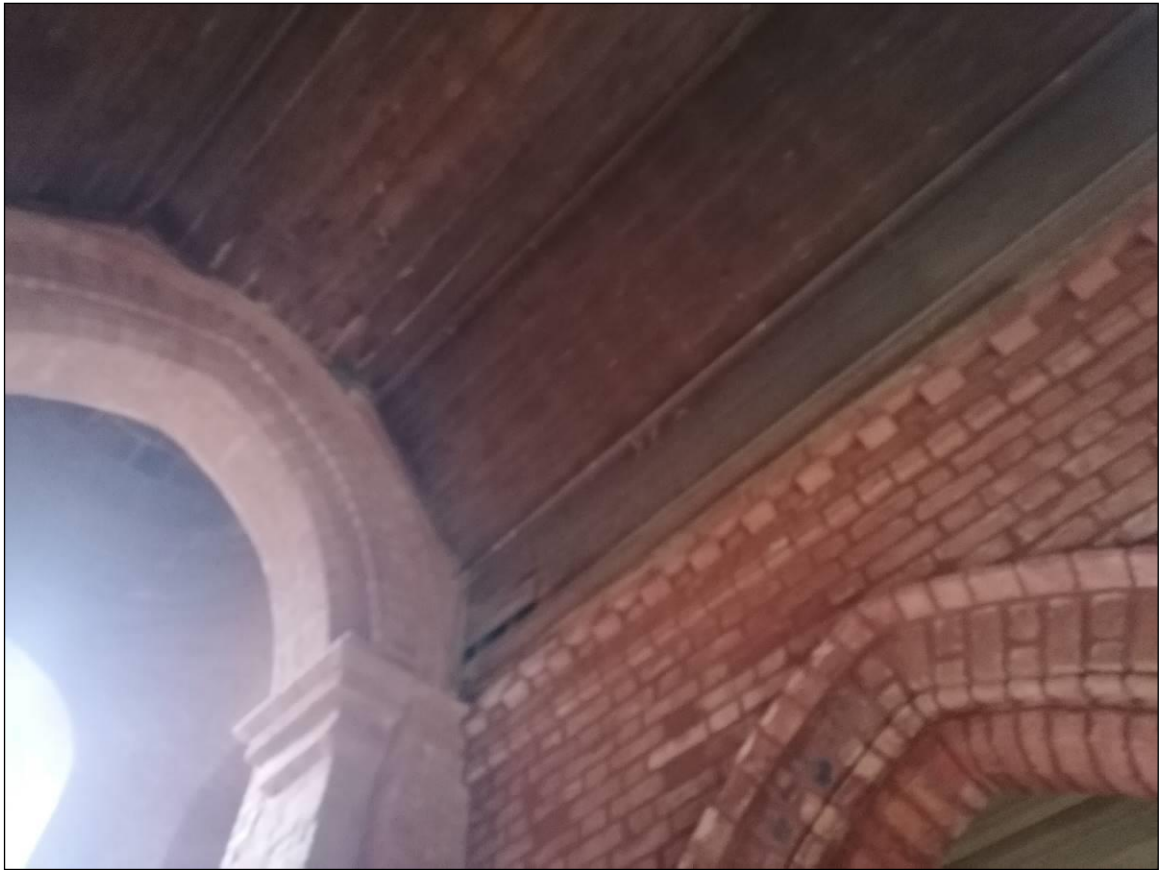
Plate 20. Original tg&v sheeting in main roof of mausoleum.
