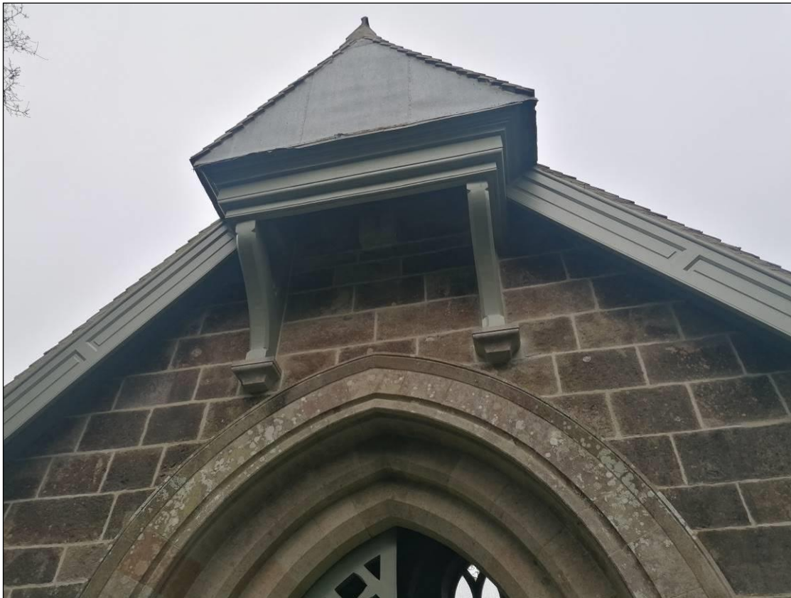
Plate 23. It is recommended that a small 18mm gap is created behind a new fascia board on the bell cote over the entrance to afford a roosting location for bats.
