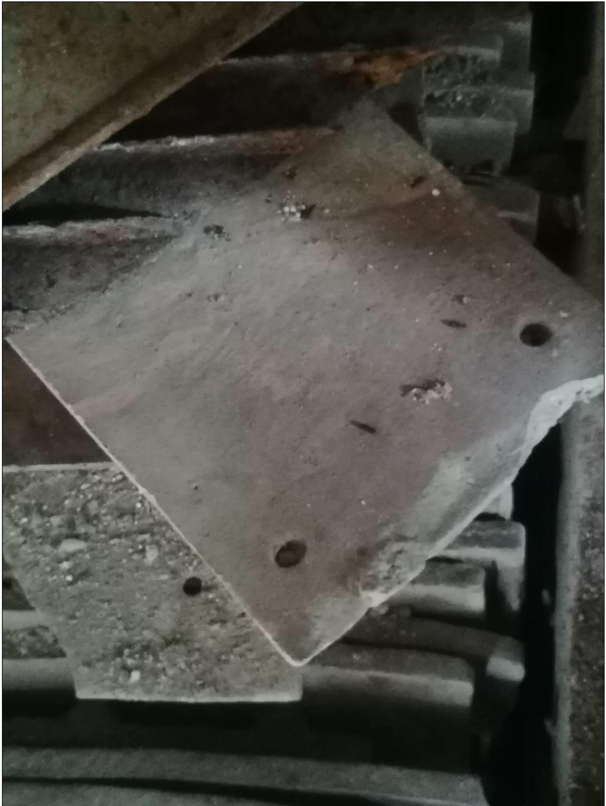
Plate 5. Old clay roof tiles within the building with bat droppings.
