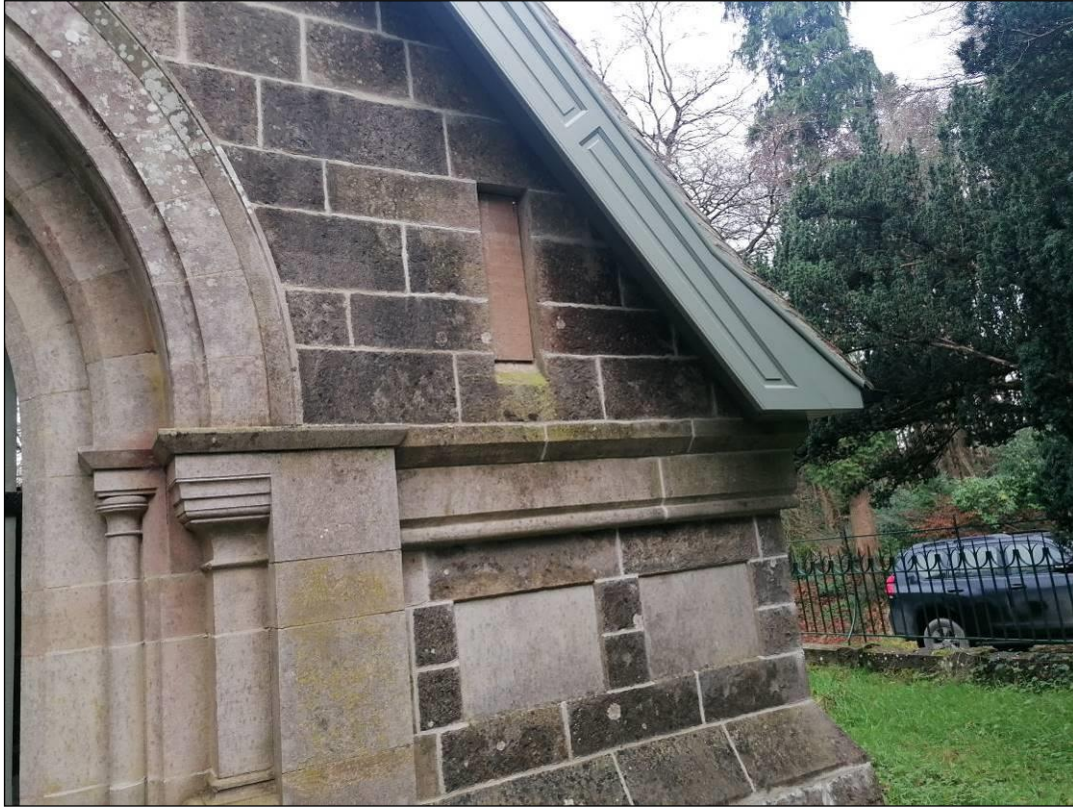
Plate 15. The window beside the door (right hand side) was also temporarily closed off but no longer provides access for bats to the mausoleum. It is recommended that a wooden louvre window is installed here.
