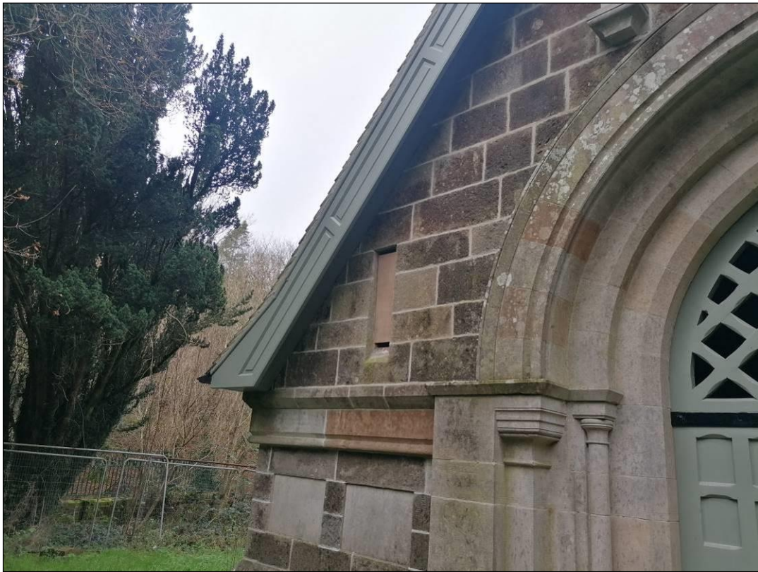
Plate 14. The window beside the door (left hand side) was temporarily closed off but continues to provide access for bats to the mausoleum. It is recommended that a wooden louvre window is installed here.
