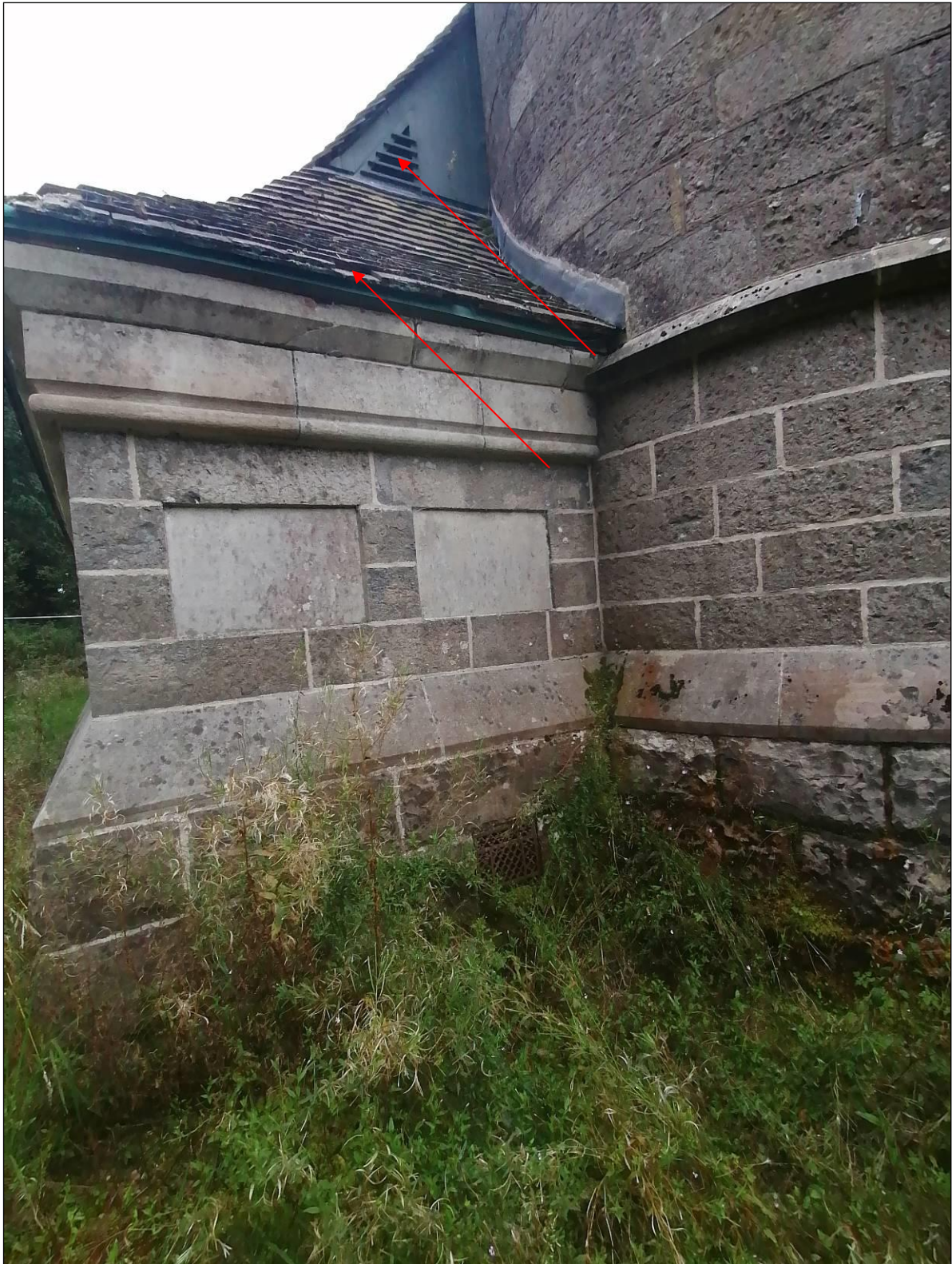
Plate 12. Gaps below clay tiles and louvered windows offer roosting potential for bats and access to the building.
