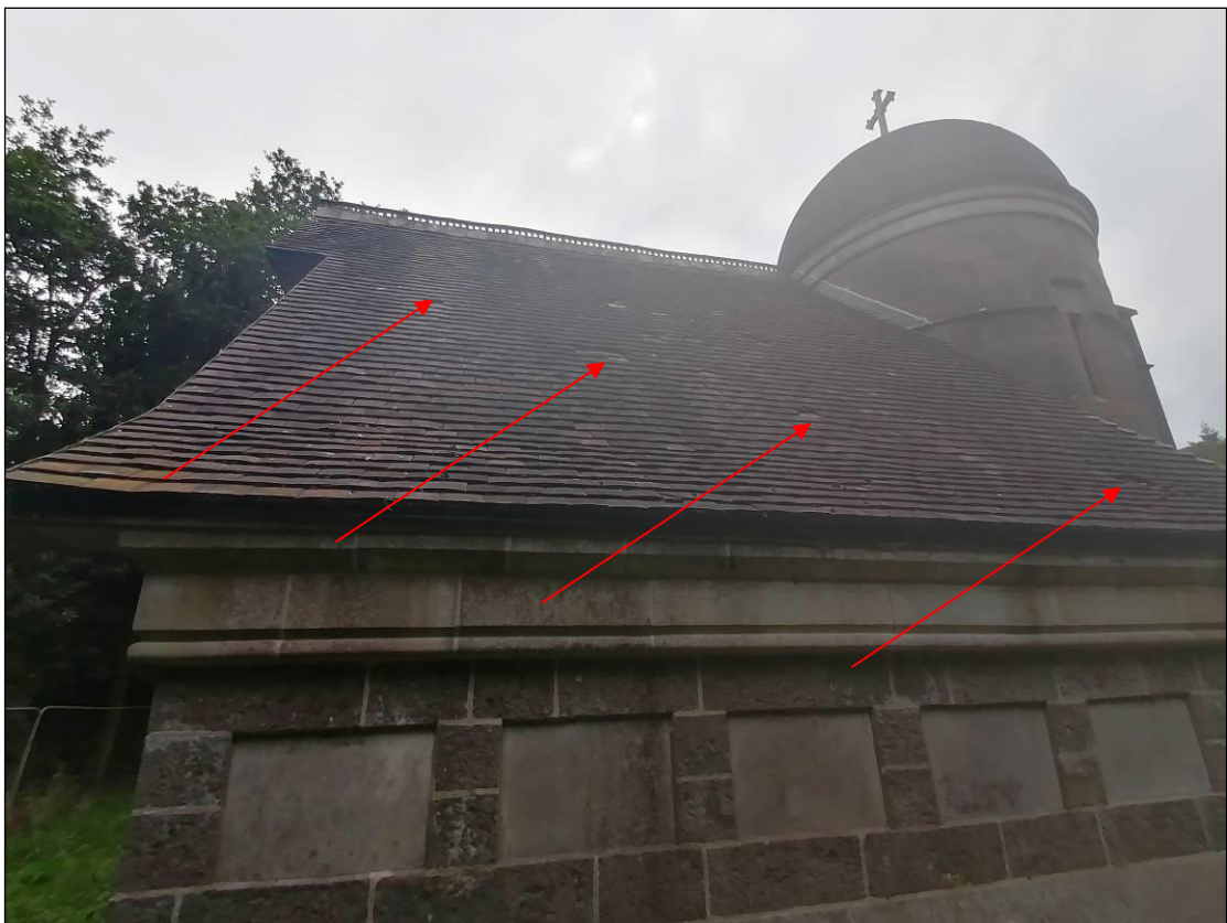
Plate 11. Slipped/missing clay tiles offer roosting potential for bats and access to the building.
