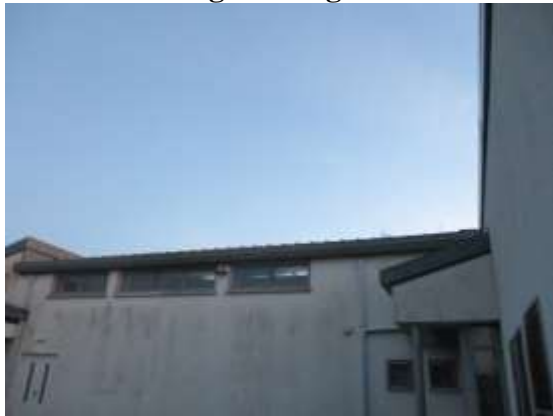
Plate 2 Roof void internally in hall showing locations where bats are entering under metal roof.
