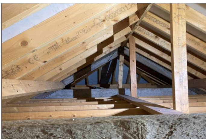
Plate 12 Loft Area above the level of the wall plate - most of the timbers were replaced after the fire (2023 surveys).
