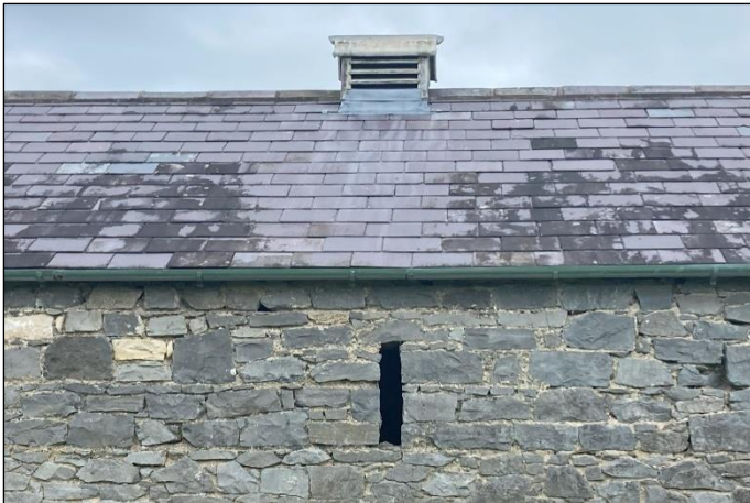
Plate 4 Louvred vent at roof apex - vertical ope and gaps in limestone wall.
