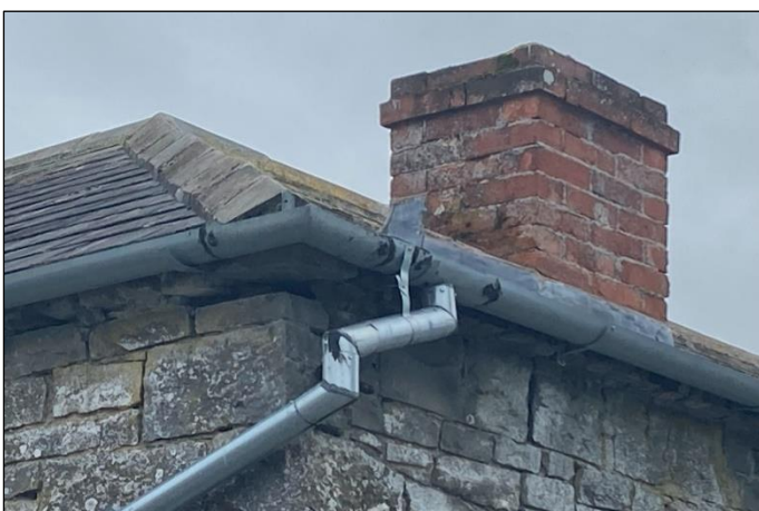
Plate 3 Corner of building - note gaps between stones.
