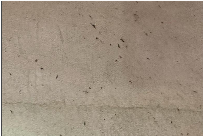
Plate 10 More bat and bird droppings on wall (2023 surveys).
