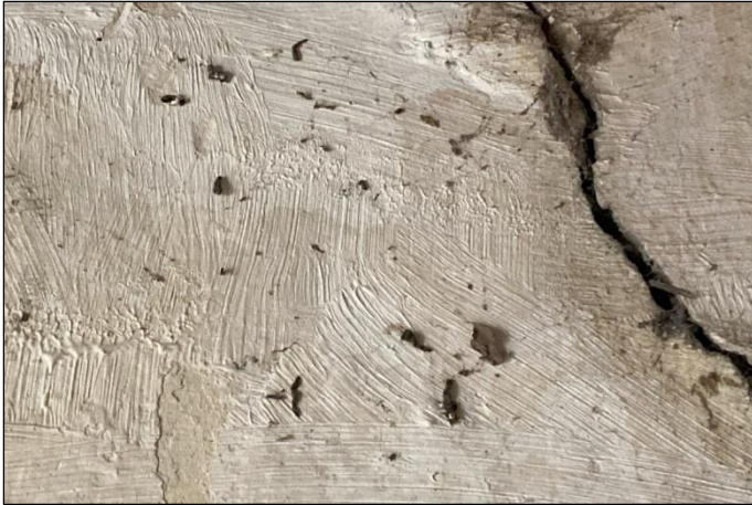
Plate 7 Bat droppings on interior rendered wall (2023 surveys).
