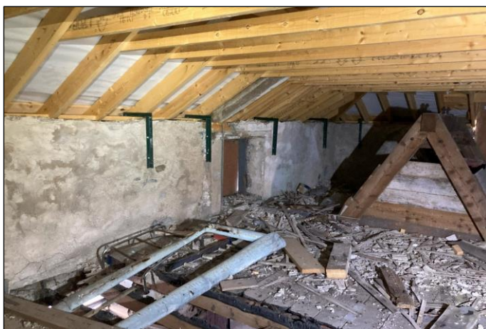
Plate 11 Loft Area - note fire damaged joists. The A-frame originally hosted a hoisting mechanism for lifting animals (2023 surveys).
