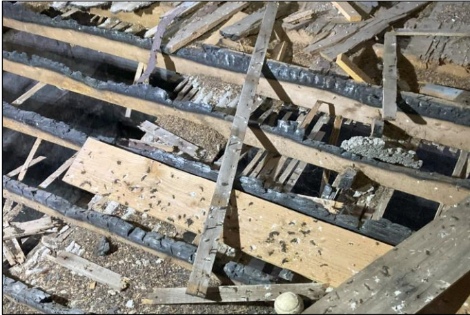
Plate 13 Loft Area - fire damaged joists and bird fouling. Bat and bird droppings present.
