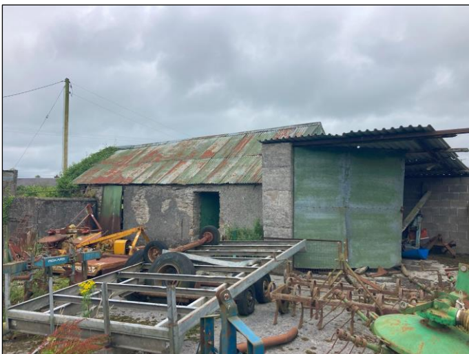
Plate 6 Front of Shed 2 - shed with green roof - bat droppings were found on interior walls, in both sections. bat droppings were found on interior walls of both sheds
