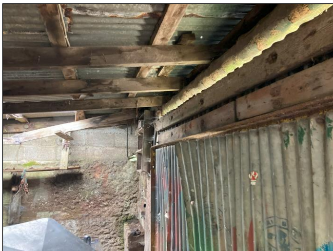
Plate 8 Interior of Shed 1 - a few bat droppings were found within. Note the arrangement of roof timbers and paucity of good bat roosts. Some of the roof covering is also missing.
