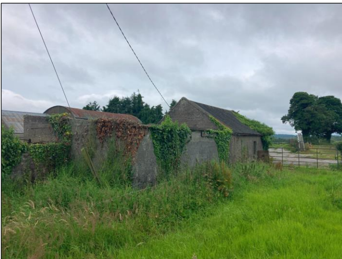
Plate 3 Rear of Shed 1 - bat droppings were found on an interior wall.
