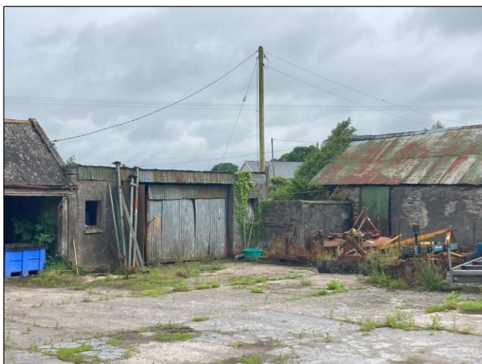
Plate 9 Sheds 1 & 3 - bat droppings were found on interior walls of both sheds.
