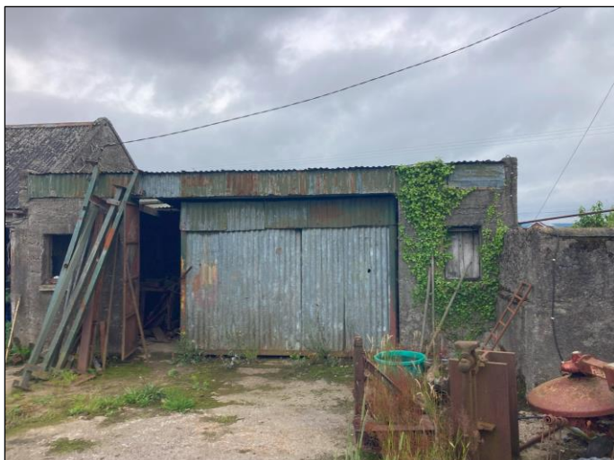
Plate 7 Front of Shed 1 - bat droppings were found within.
