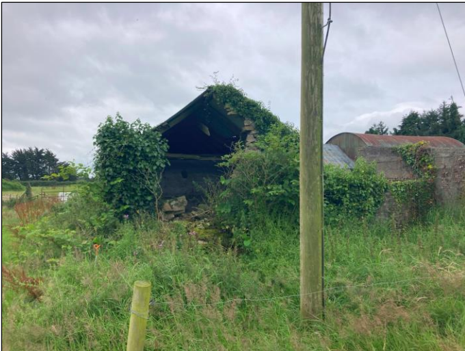
Plate 2 Rear of Shed 2 - bat droppings were found on an interior wall - note Japanese knotweed in front of shed.
