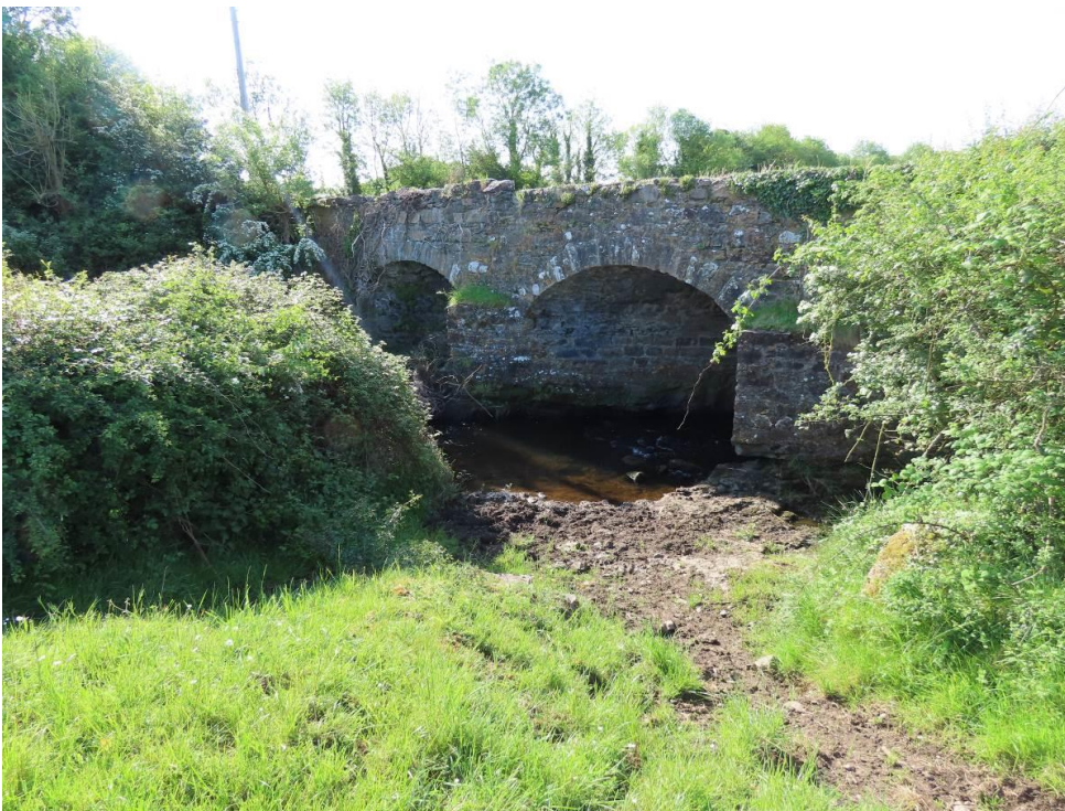
Photo 4 – upstream elevation of Duniry 2 Bridge. The westernmost arch is obscured by vegetation
