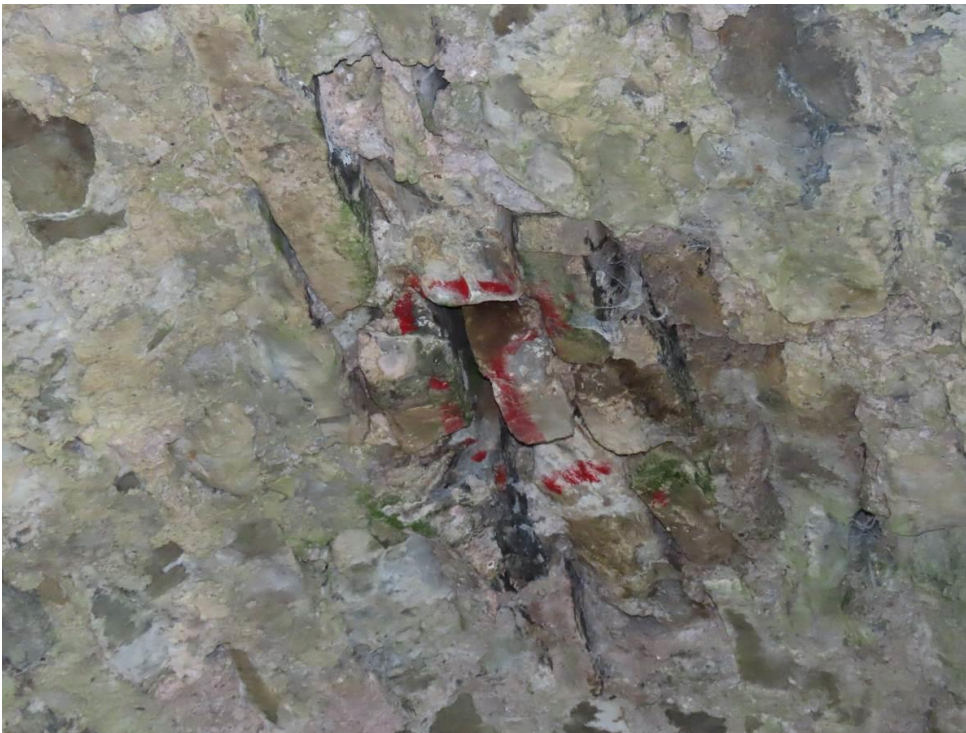
Photo 14 – close up of void containing maternity roost. This void must be retained
