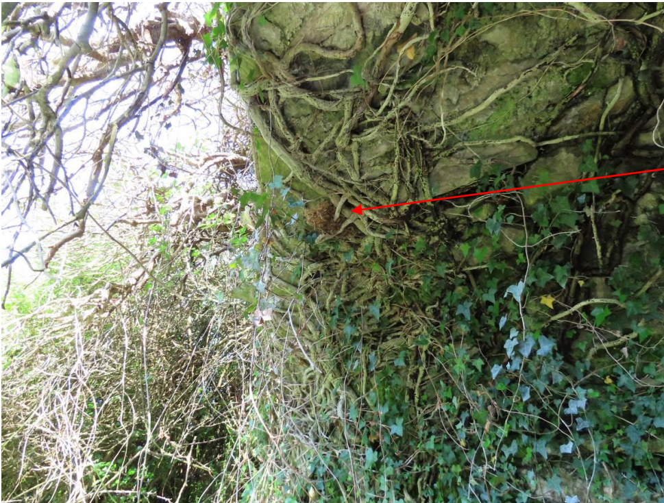
Photo 8 – wren's nest in ivy at upstream face of arch 1
