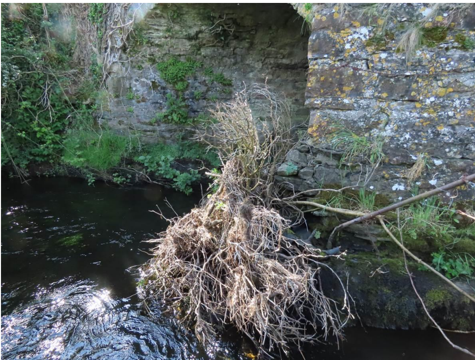
Photo 12 – flood debris trapped at upstream pier between middle arch and eastern arch
