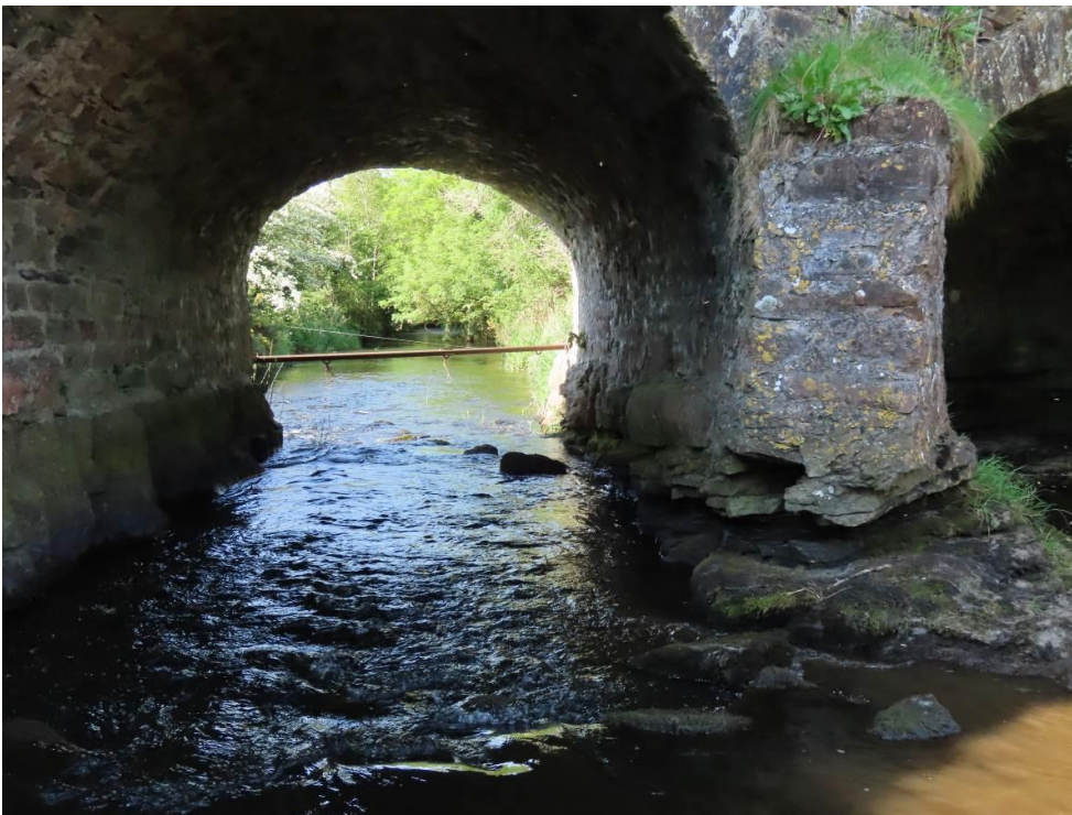
Photo 10 – upstream face of middle arch and western arch. Breakwater pier undermined
