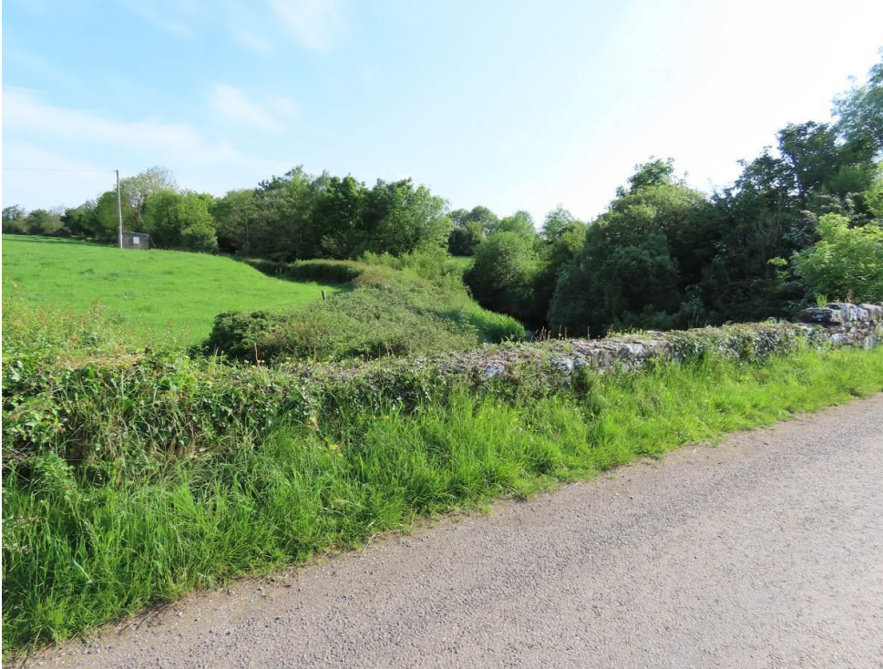
Photo 3 – upstream parapet wall with heavy vegetation
