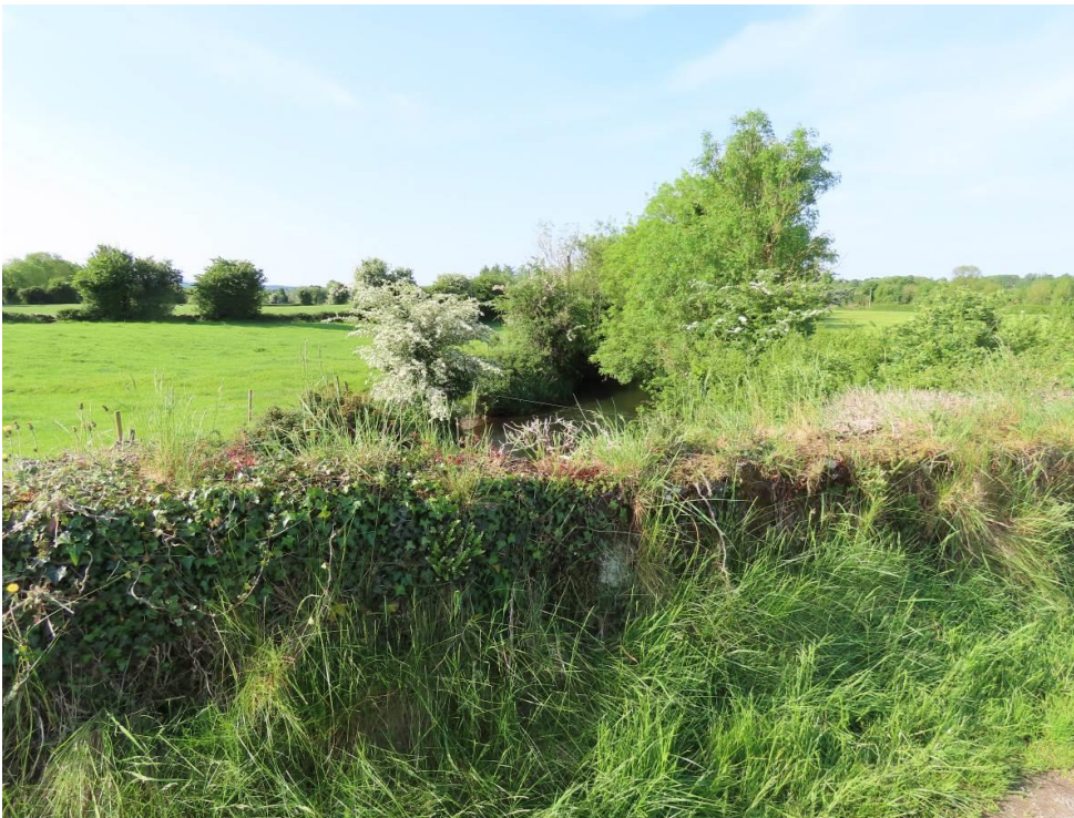
Photo 2 - downstream. Parapet wall heavily overgrown with vegetation
