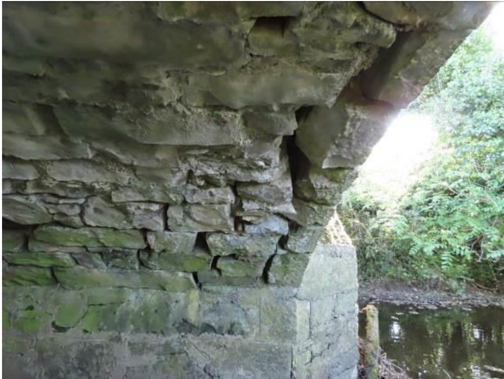
Photo 45 – crack behind facing stones of Arch 2
