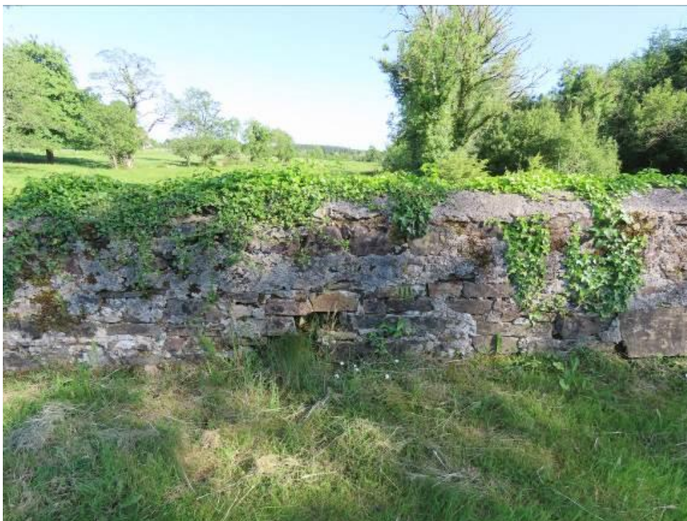
Photo 40 – damaged parapet wall
