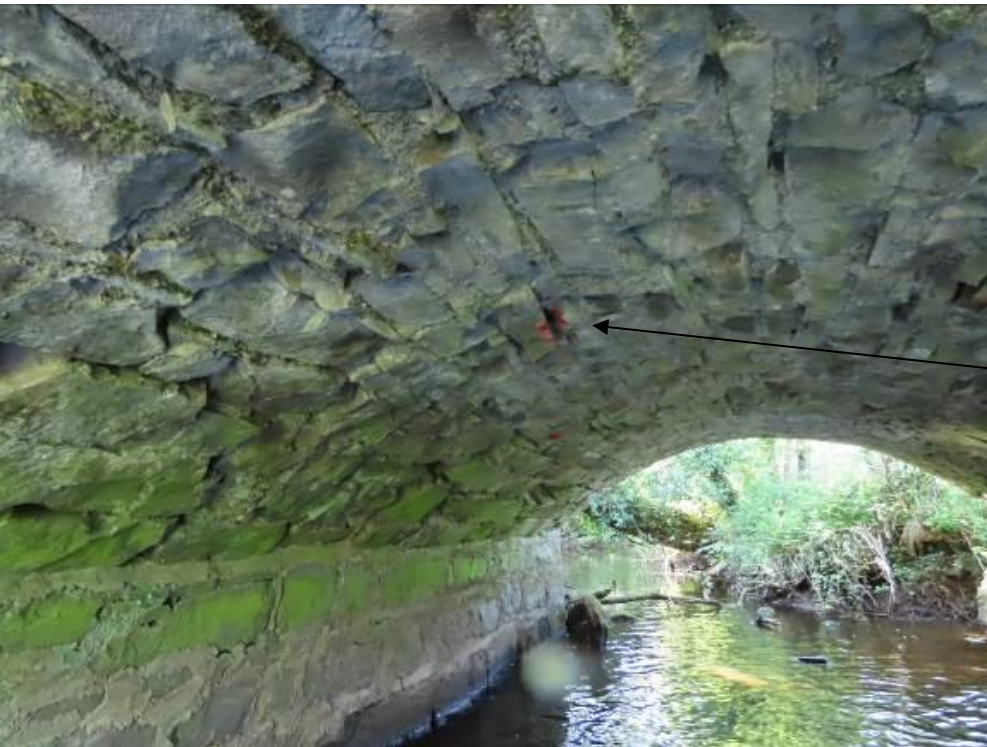
Photo 48 – crevice containing single Daubenton's bat under Arch 4
