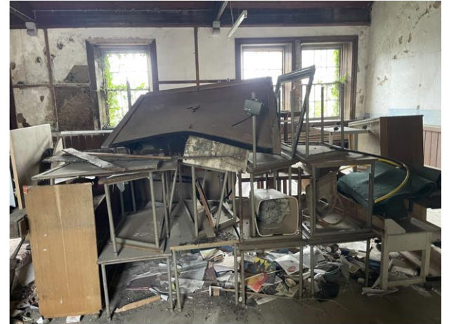
Plate 6: Internal view of upper floor of former school house with bat detector installed. High daytime light levels
