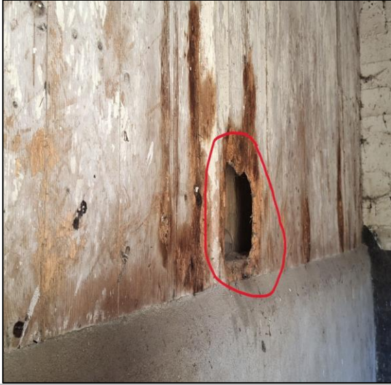
Plate 19: An access point into the cavity of a wooden partition in the stables in S07
