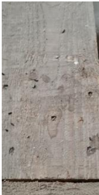
Bat droppings on pallet; building 3
