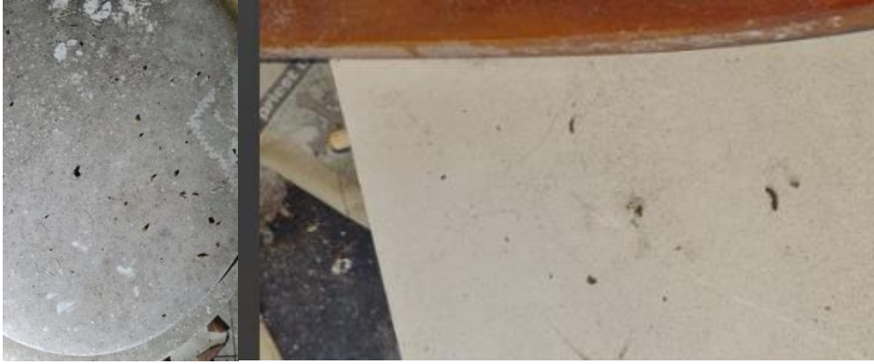
Bat droppings – building 11
