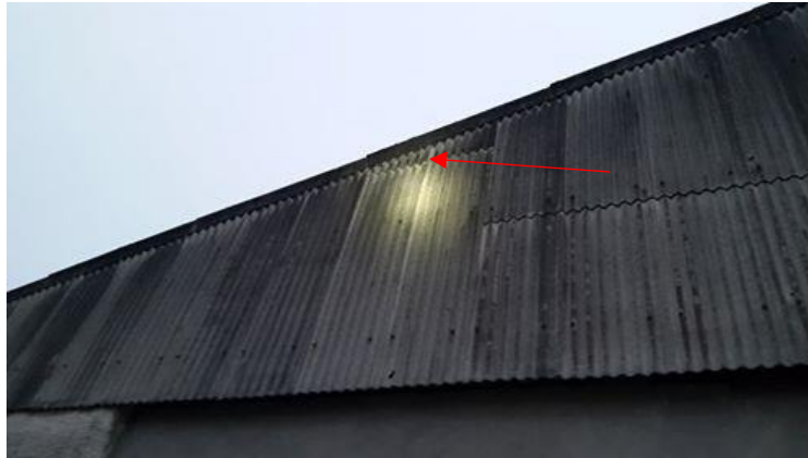
Roost area under asbestos join, building 3
