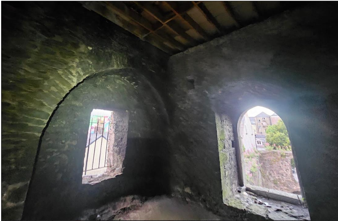
Plate 9. Windows in the tower are covered with a 1cm grating to prevent access by birds. This also limits bat access to roosting spaces within the tower.
