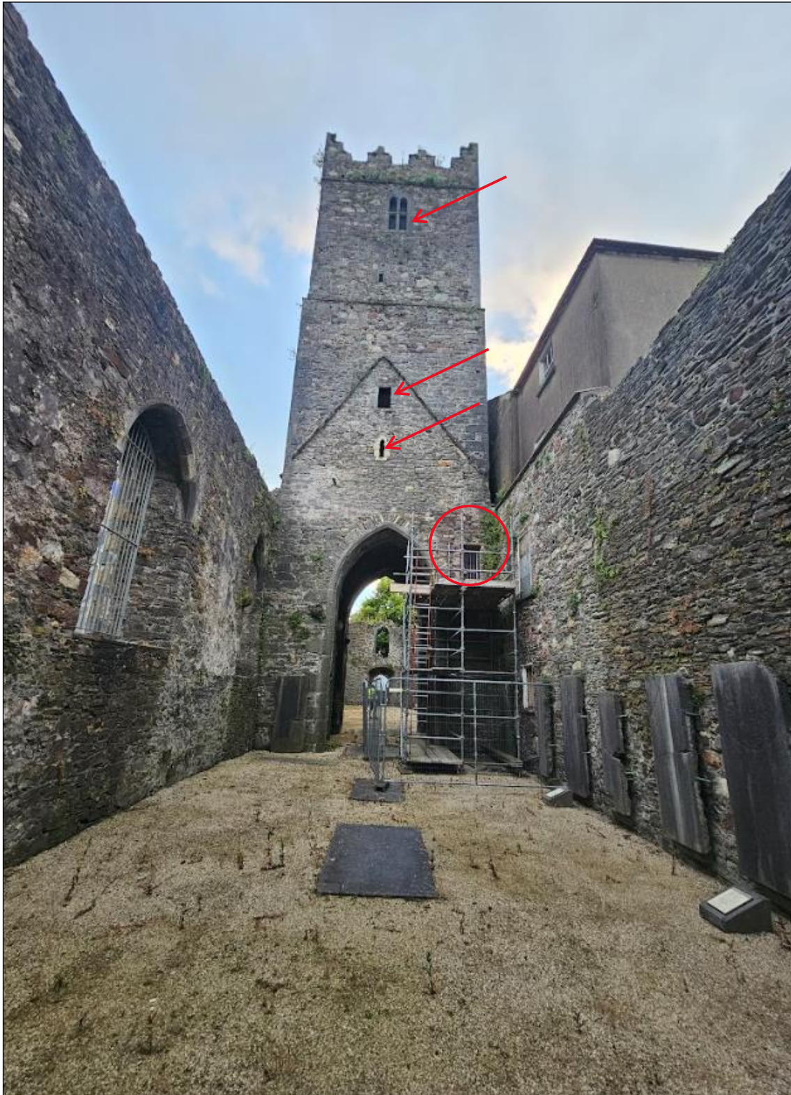
Plate 15. Level 0, showing the length of the chancel, the transept and tower with the nave and entrance beyond. The red arrows highlight openings that provide potential access points for bats, if the grating is appropriately modified. Access door circled in red.
