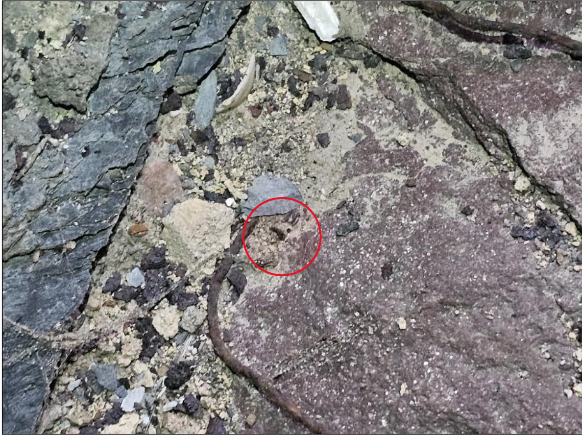
Plate 5. Bat droppings found in on the window sill (circled in red).
