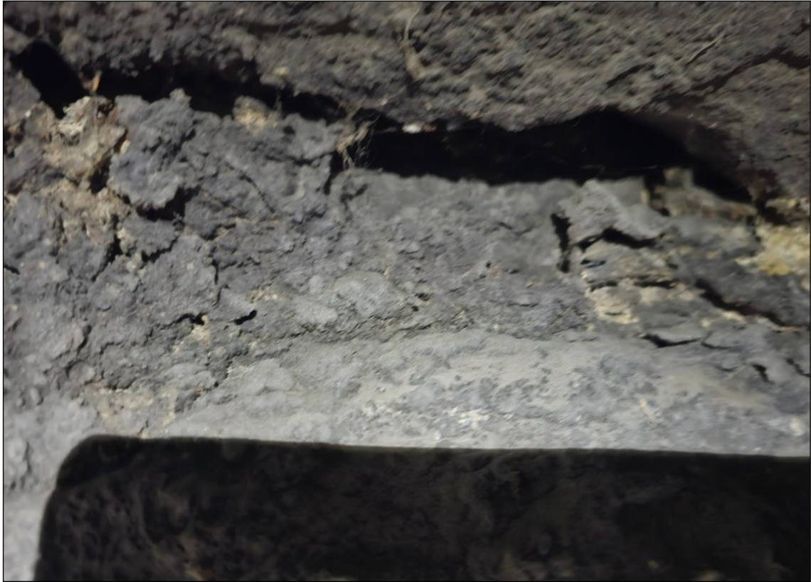
Plate 7. Tower walls above the windows. Note the crevices and ledges in the rough mortar finish, providing bat roosting shelter in the walls and stonework.
