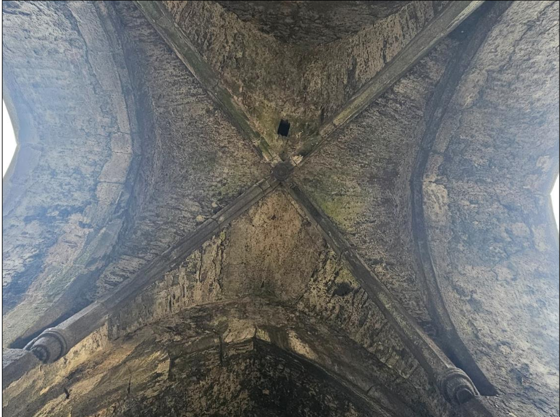
Plate 6. Level 0, Transept archway. There are many suitable locations in the stonework here that bats could avail of for roosting purposes.
