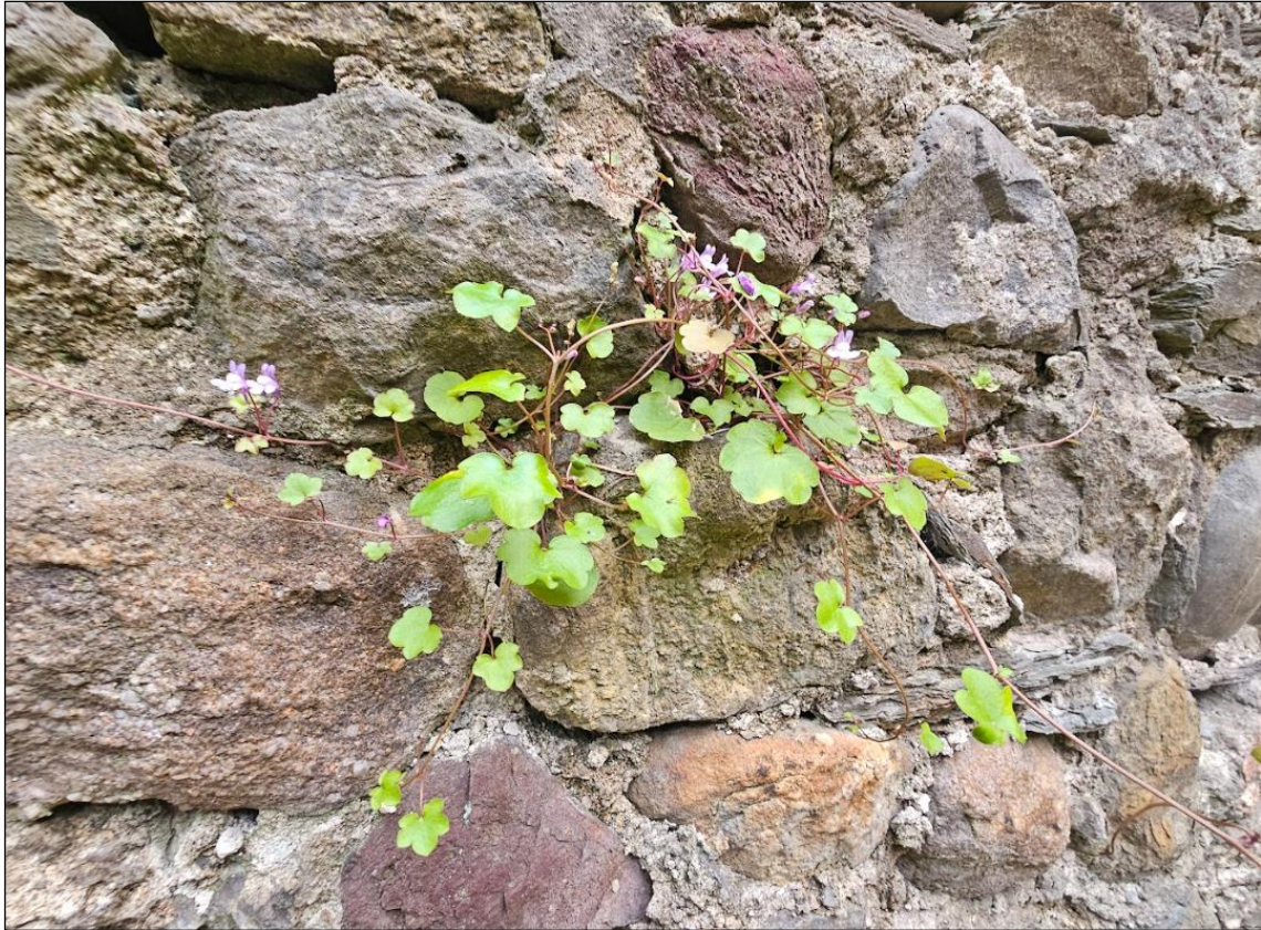
Plate 21. Some areas of the walls have significant vegetation such as this cover of ivy leaved toadflax. Vegetation such as this does not compromise the building in comparison to species such as trees and dense ivy whose roots can work their way into the wall structure.
