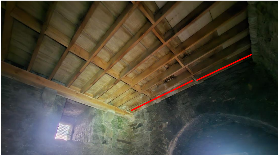
Plate 17. Level XX, showing a covered ceiling with exposed joists. This provides safe roosting opportunities for bats, without risk of entanglement in roofing membranes. Timbers here can be doubled up to create a roosting location for bats – indicative locations for timbers shown by red line.
