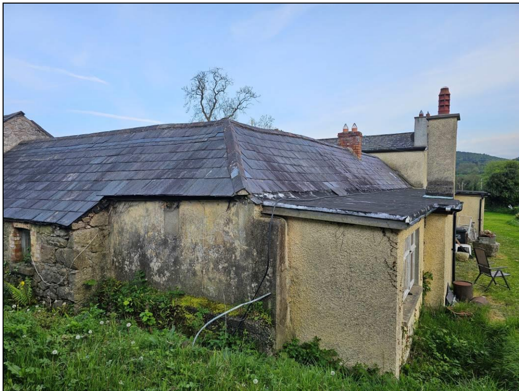
Plate 10. Looking south over the flat roof extension adjoining The 'Games Room', 'File Storage Room' and 'Office'.
