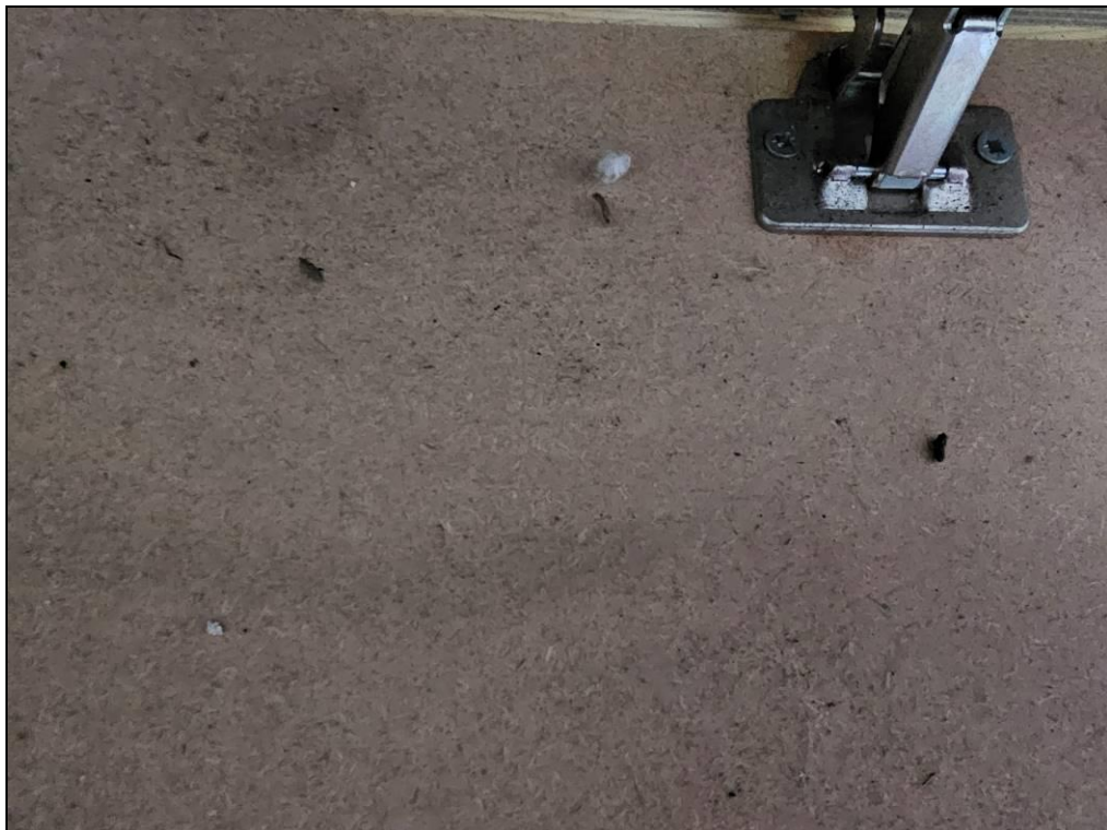
Plate 2. Bat droppings on the attic hatch in the main house.
