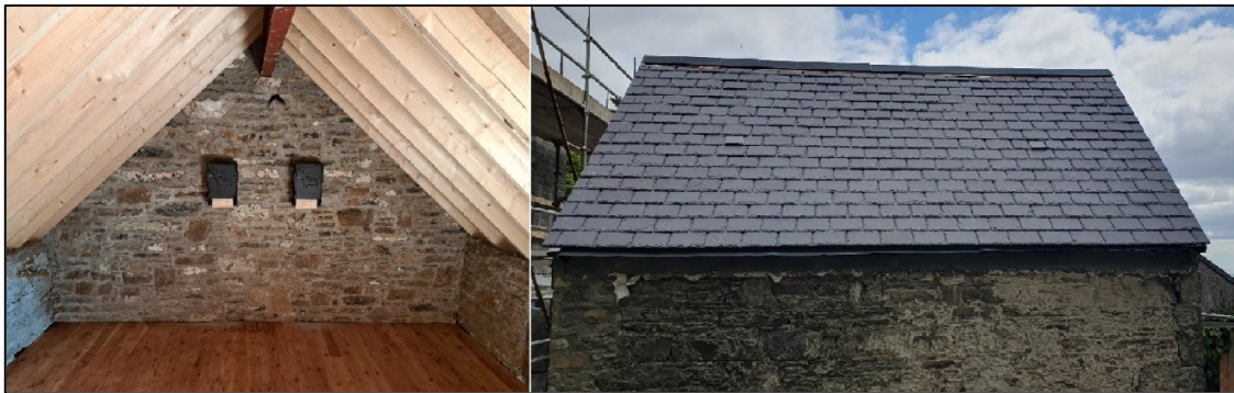
Plate 3: Internal area of dedicated bat roosting loft showing rafter roost crevice timbers & bat boxes (left) and western roof slope with 2 x bat access slates (right).
