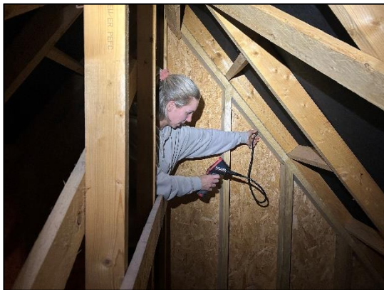
Plate C. Internal inspection in search of a Pipistrelle maternity roost within the attic of a property in Cork.
