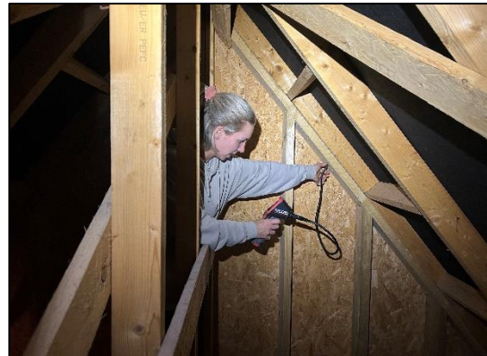
Plate D. Internal inspection in search of a Pipistrelle maternity roost within the attic of a property in Cork.
