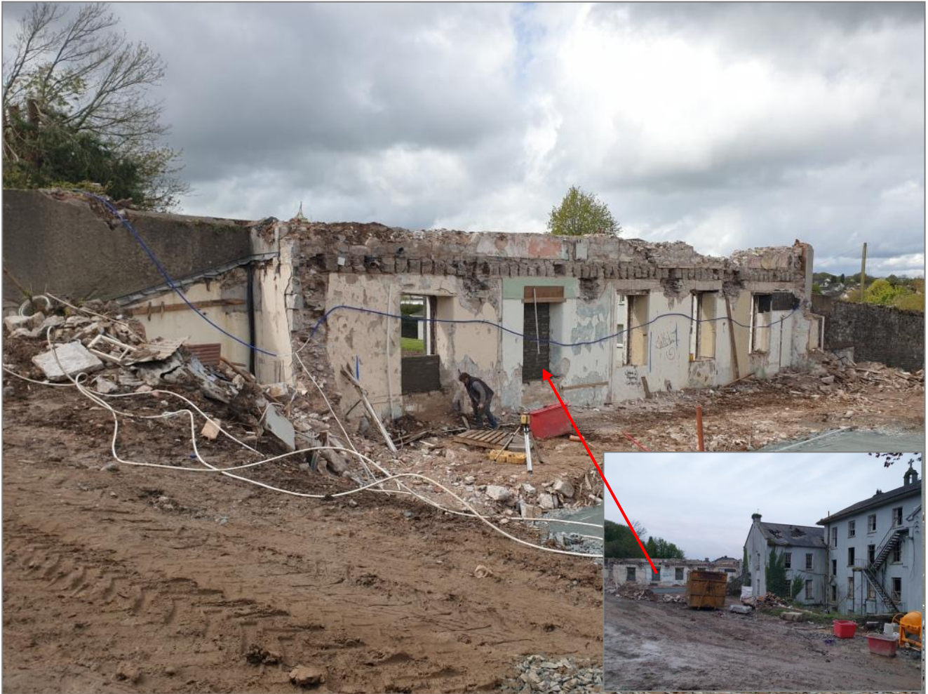
Plate 6. Remaining wall of the former nursing home wing that was at the SE corner of the convent building (inset).
