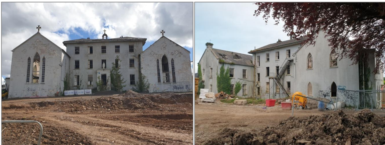
Plate 1. Photographs of the front (left) and rear (right) of the former Presentation Convent Mitchelstown.
