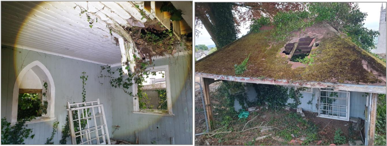
Plate 8. Low bat roost potential and no signs of bat roosting in this gazebo structure
