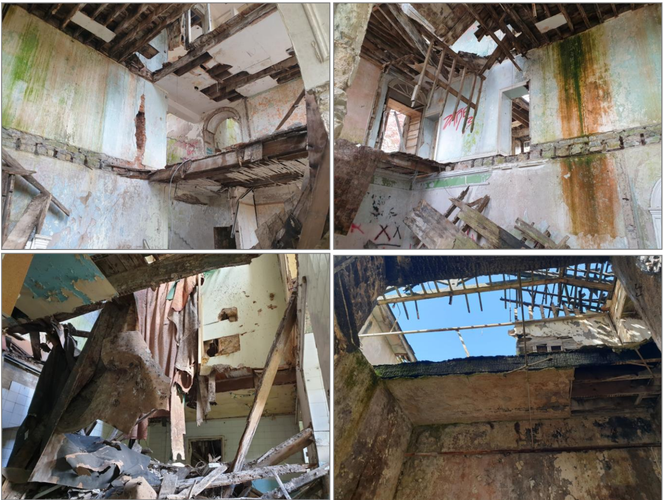
Plate 5. Photographs showing fire damage, and collapsing floors, ceilings and roof of the former convent building
