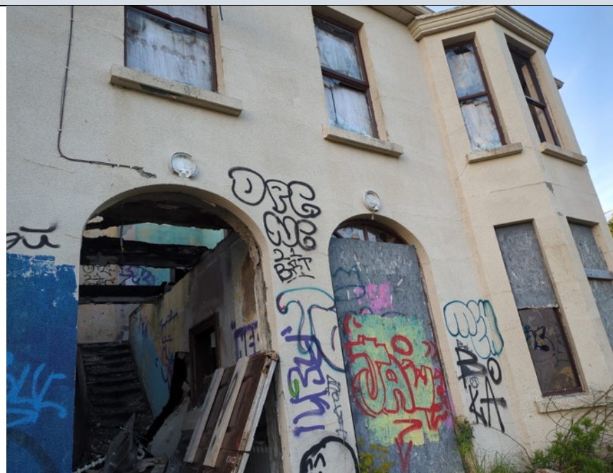
Plate 2. Windows and doors open with graffiti evident.
