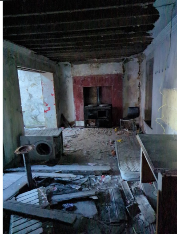
Plate 5. Interior room in poor condition
