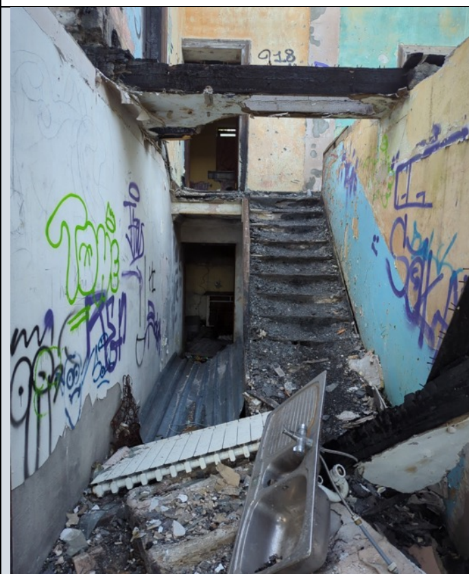
Plate 4. Interior to front. Badly fire damaged.
