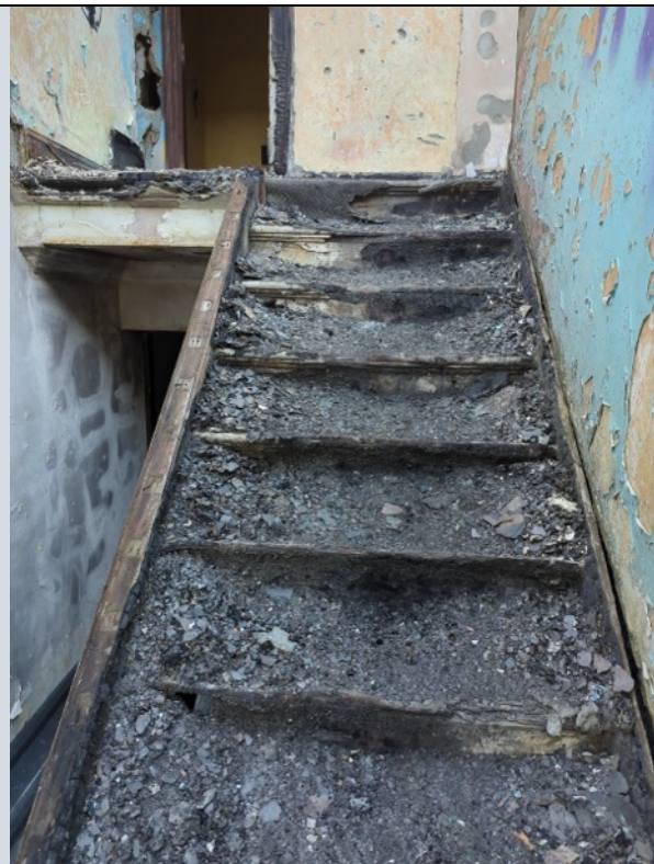
Plate 6. Stairs badly fire damaged and in dangerous condition
