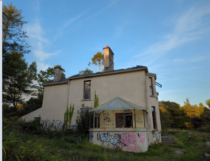
Plate 1. Western gable with windows broken
