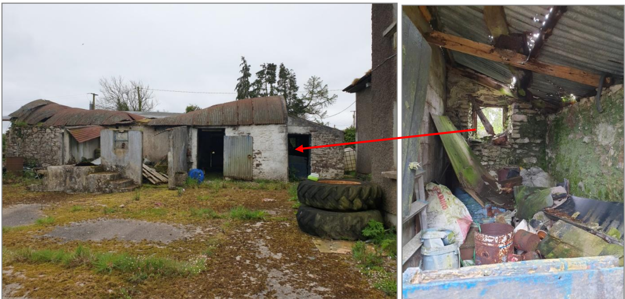
Plate 13. Small section of stone shed with a slanting roof where alternative bat roost spaces to be created
