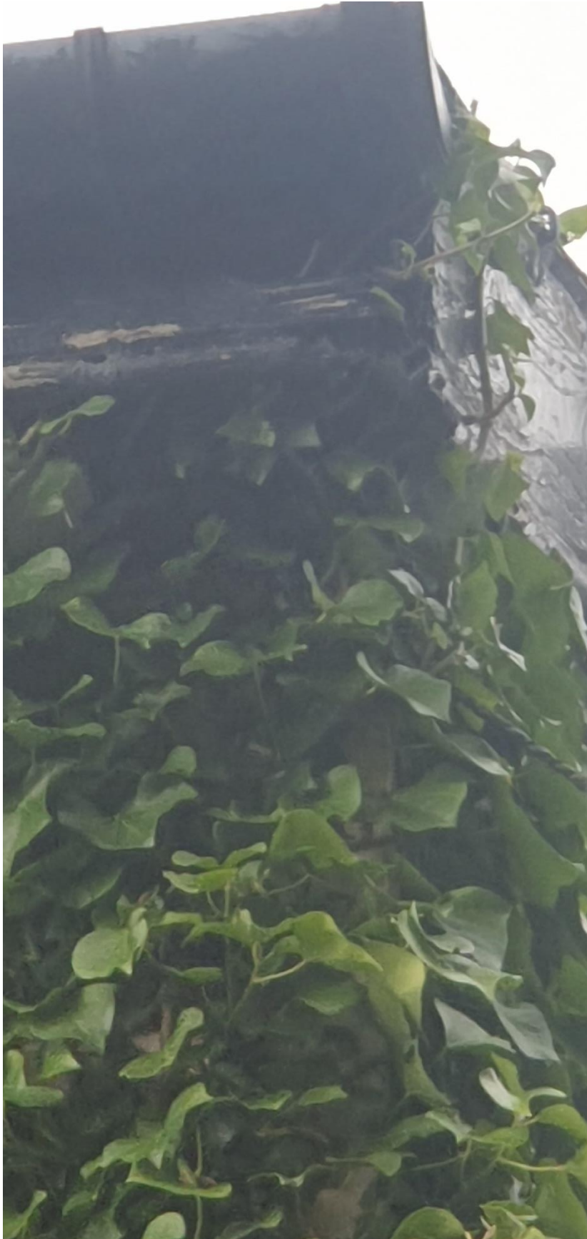
Photo 6. Close-up of eastern corner of house where NPWS and KCC recorded a bat roost, was not occupied for this survey - possible entrance where fascia has rotted
