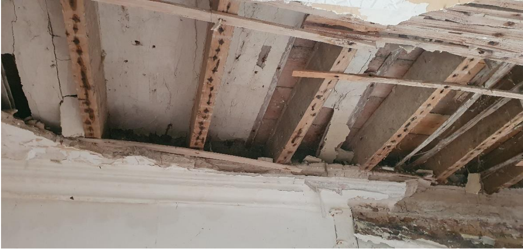
Photo 1. Example of where ceiling has fallen down providing potential space for bats between ceiling and the floor
