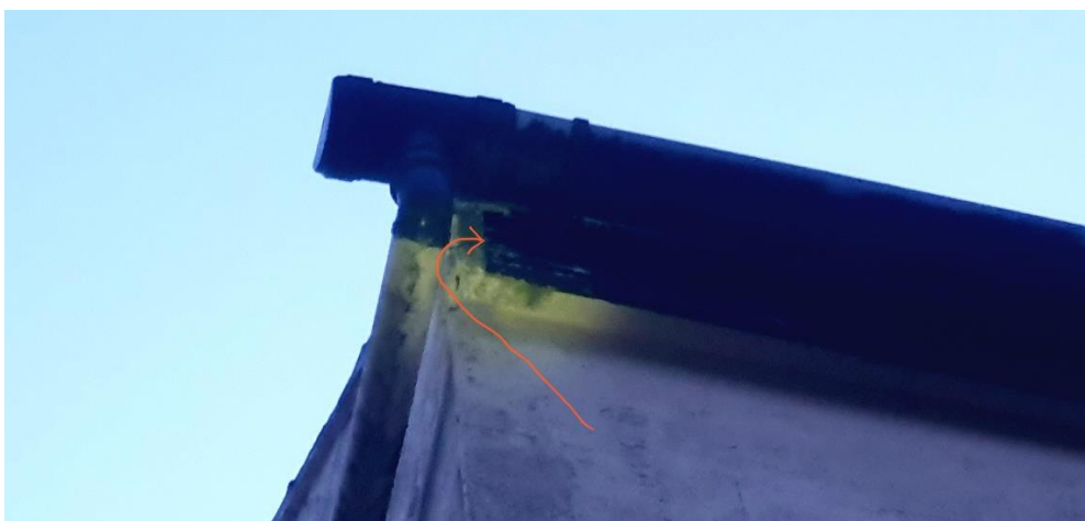
Figure 9. Arrow indicates where bats climb under the fascia
