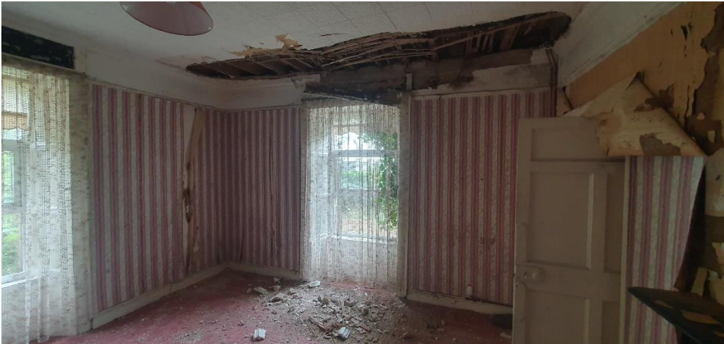
Photo 2. However, there was no evidence of a potential pathway for bats to enter from the outside. House in serious disrepair
