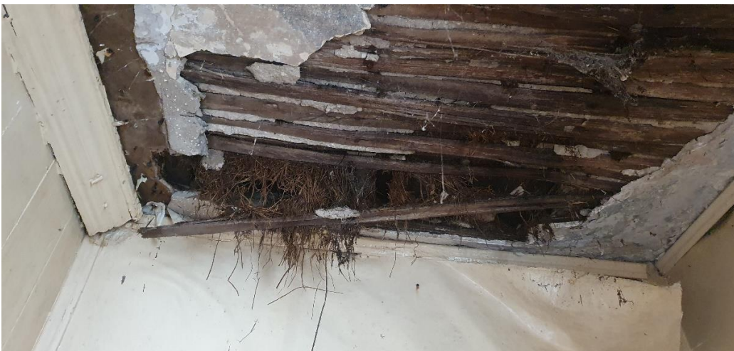
Photo 3. Roots of vegetation breaking through the ceiling of the basement
