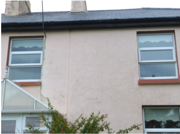
Photo 1: Front of house with uPVC windows, cracking in wall plaster and rotting fascia/soffit
