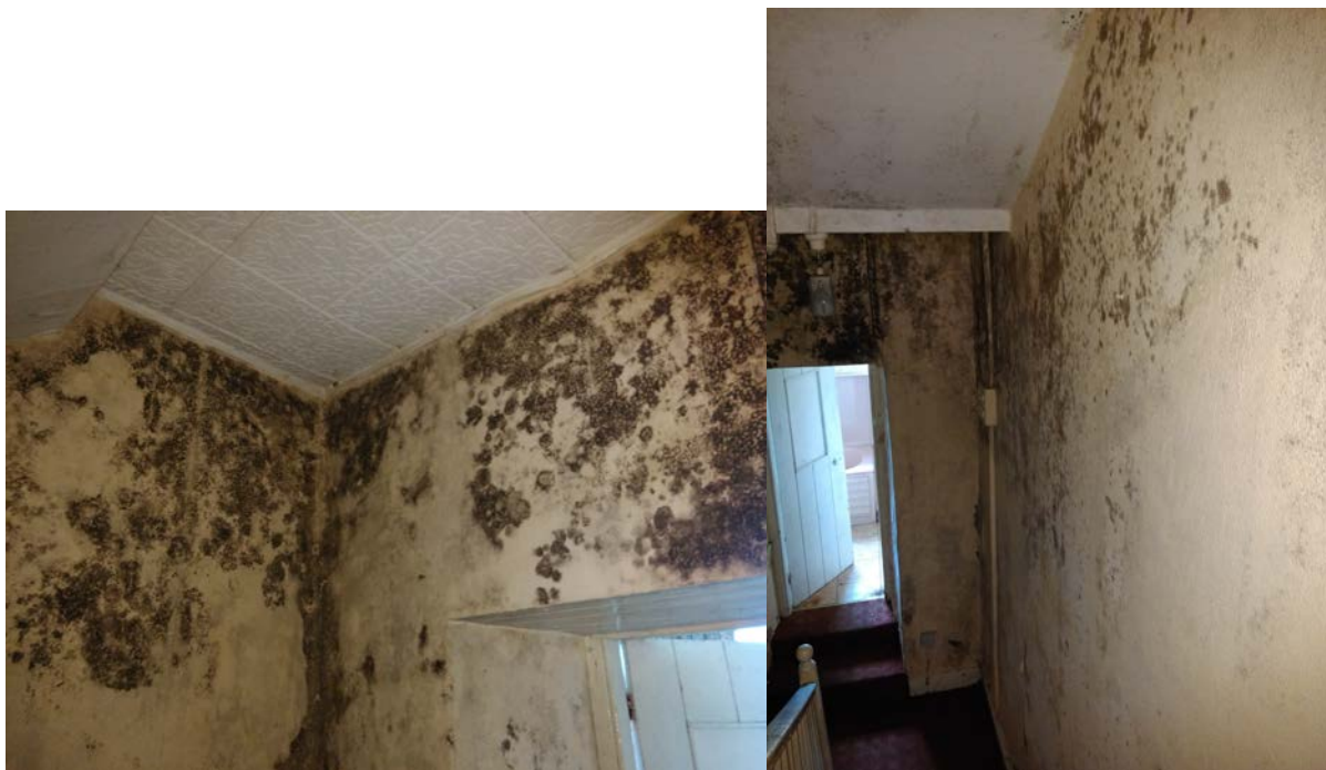
Photos 24 & 25: Mould and damp in the stairwell
