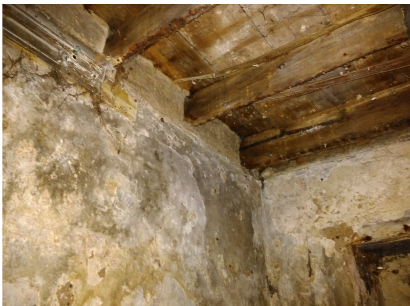
Photo 15: Rotting timber trusses and further evidence of deterioration in the walls
