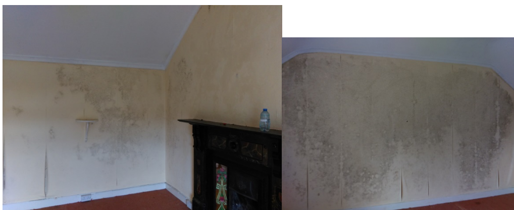
Photos 32 & 33: Further damp and mould on first floor
