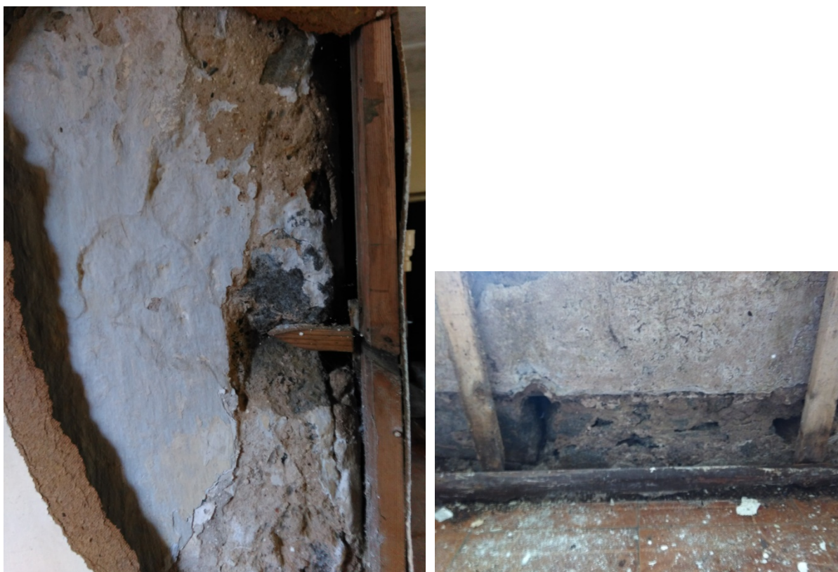
Photos 13 & 14: Evidence of sea gravel used in mortar, spalling and deterioration in the mortar
