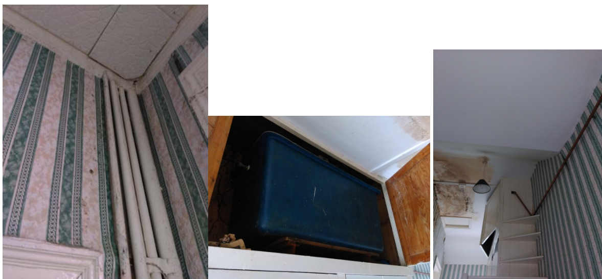
Photos 36, 37 & 38: Exposed plumbing and water tank in a press at top of stairs
