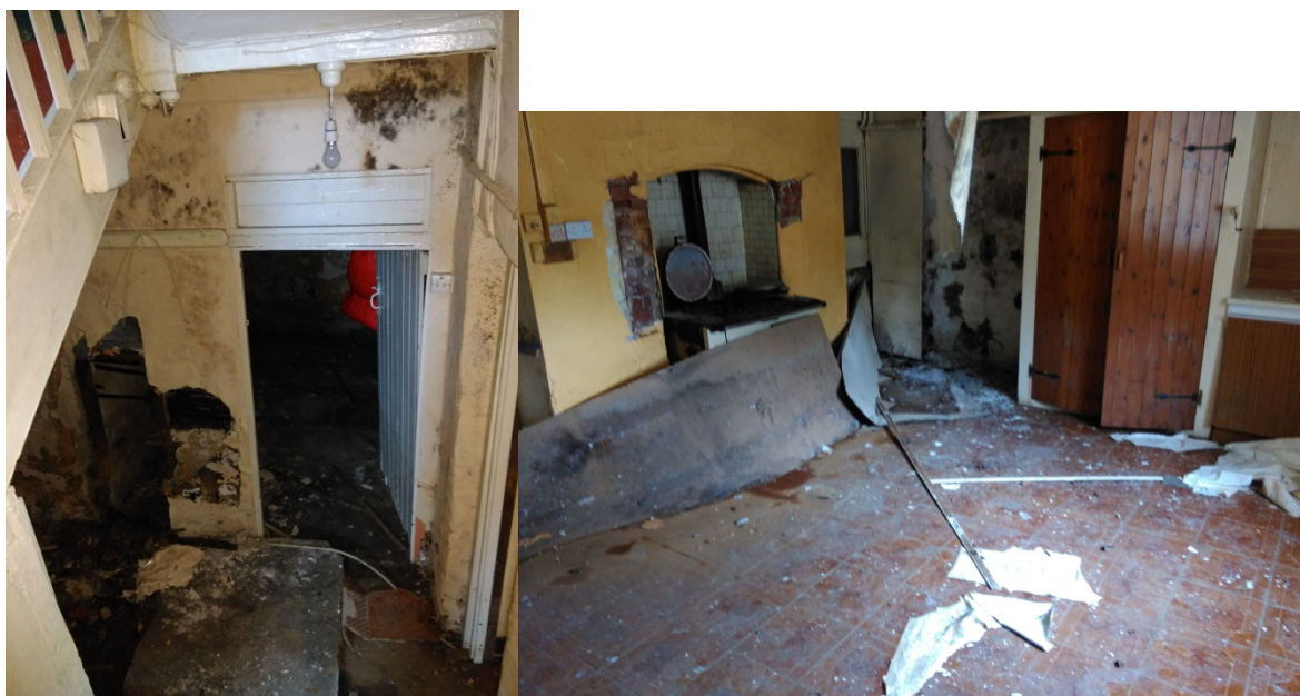
Photos 28 & 29: Basement with significant mould, dampness and water damage
