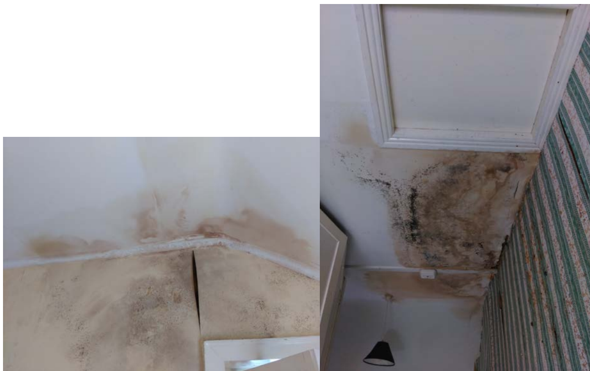
Photos 34 & 35: Evidence of water ingress and damage through the roof/ceiling
