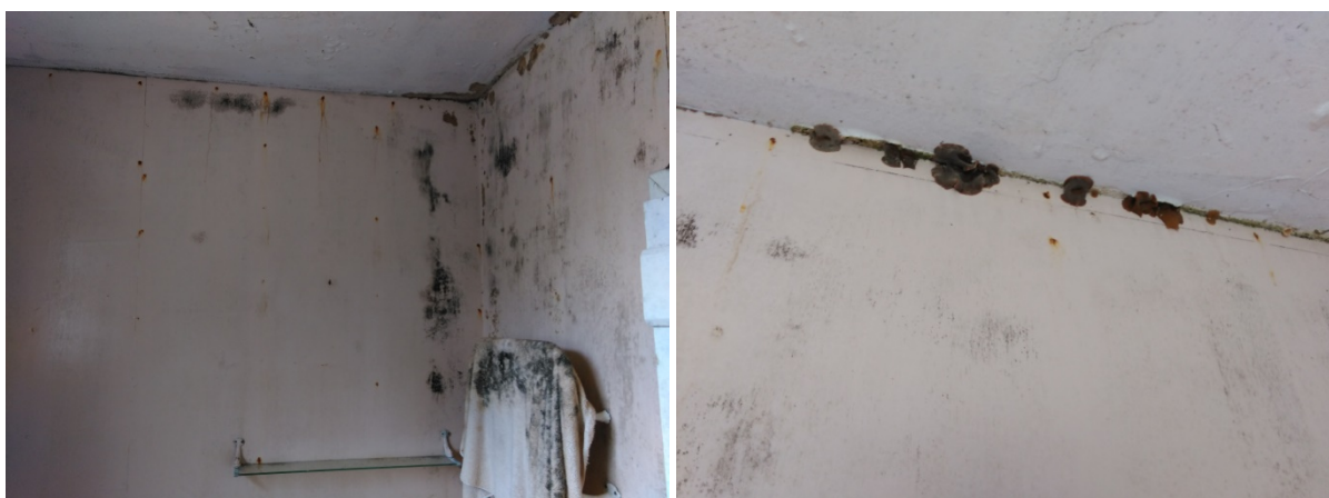
Photos 30 & 31: Further damp and mould in bathroom with growth of fungus
