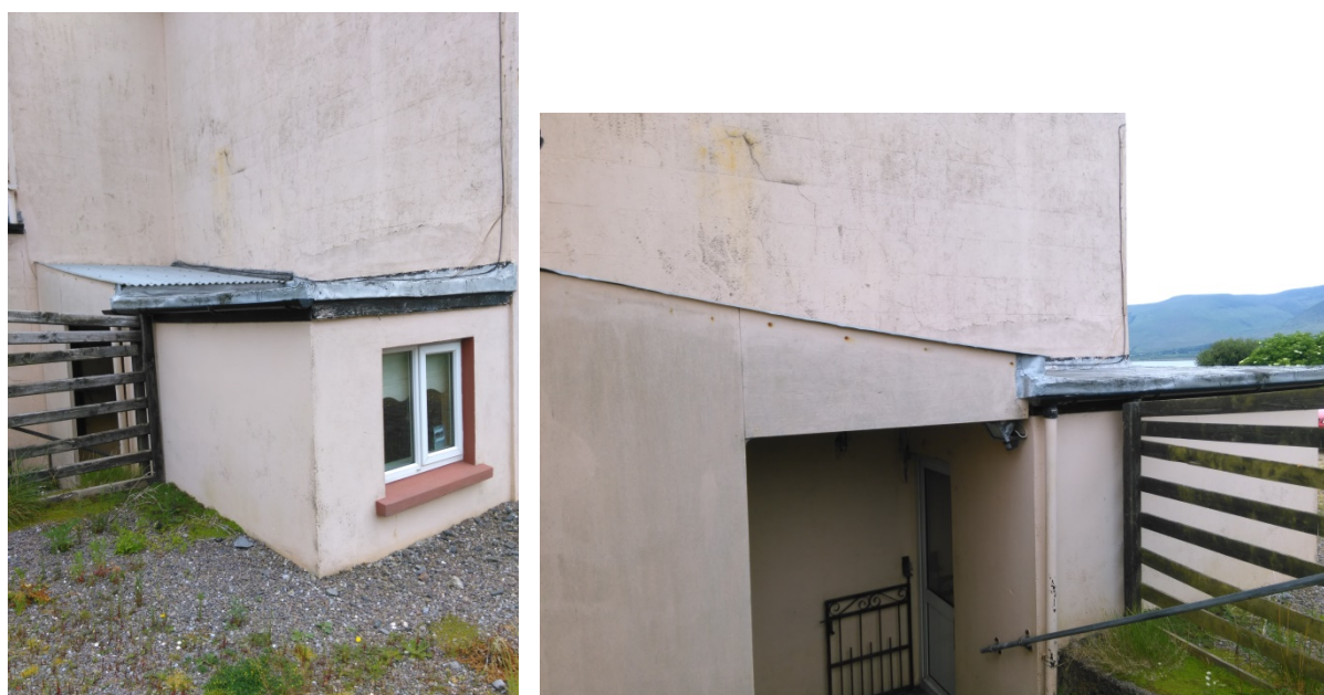
Photos 7 & 8: Poor quality extension and significant crack on wall
