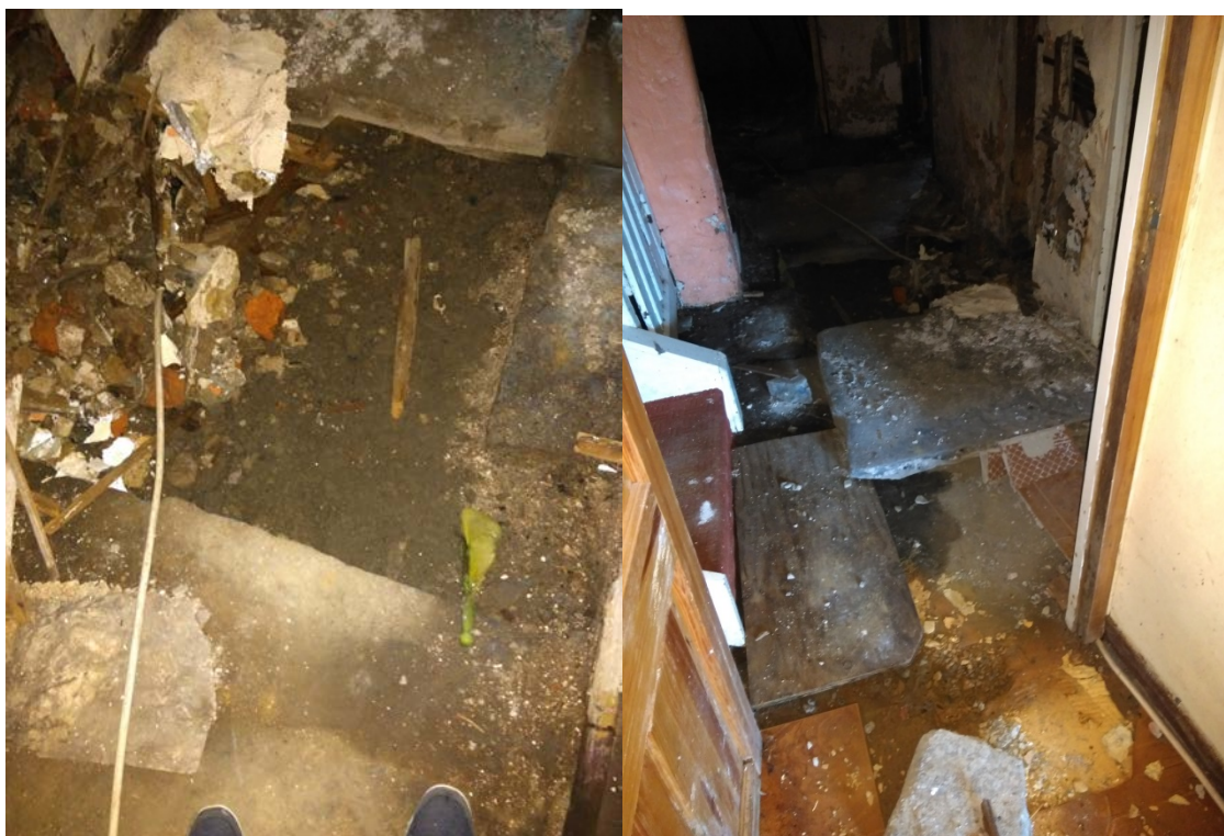
Photos 20 & 21: Excavation of floor to show earth foundation and evidence of flooding damage
