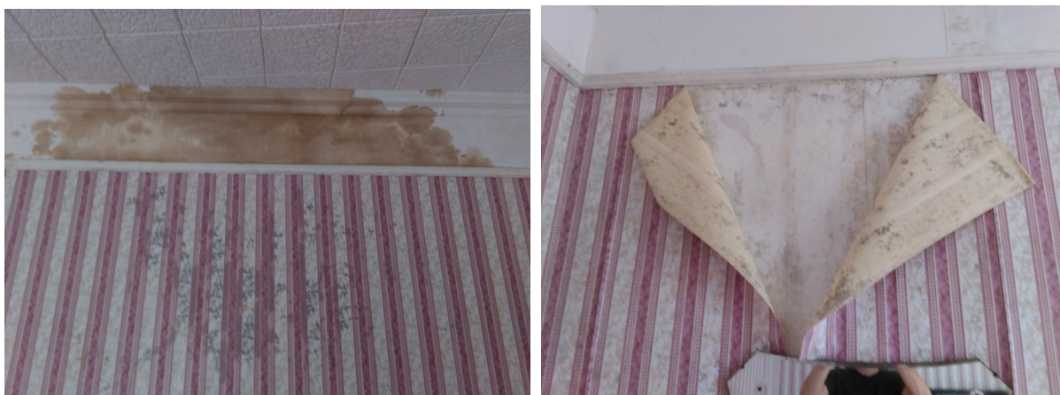
Photos 26 & 27: Mould and damp penetrating the plastic/Styrofoam and wallpaper wall covering and wallpaper peeled back to show Styrofoam covering (ground floor)
