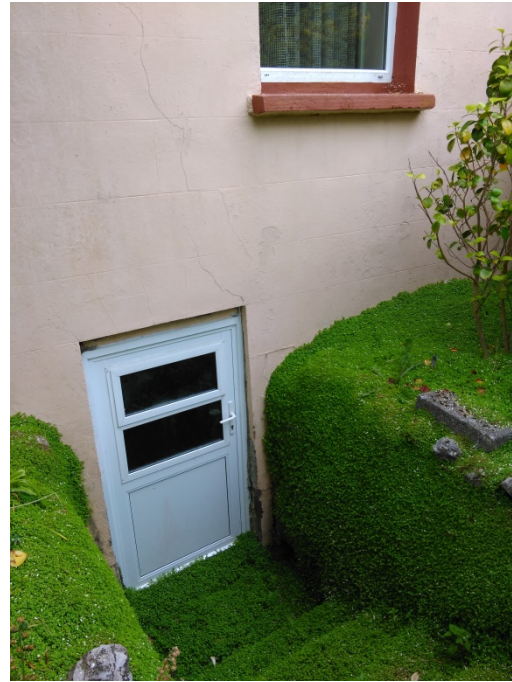
Photo 2: Basement entrance with significant cracking on wall and growth of mosses
