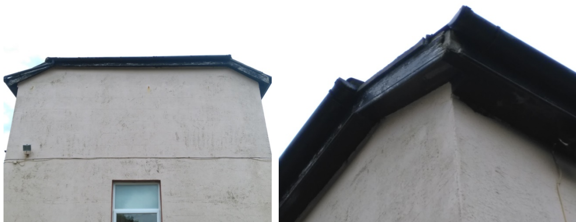
Photos 5 & 6: Side of house with significant plaster cracking and rotting fascia/soffit
