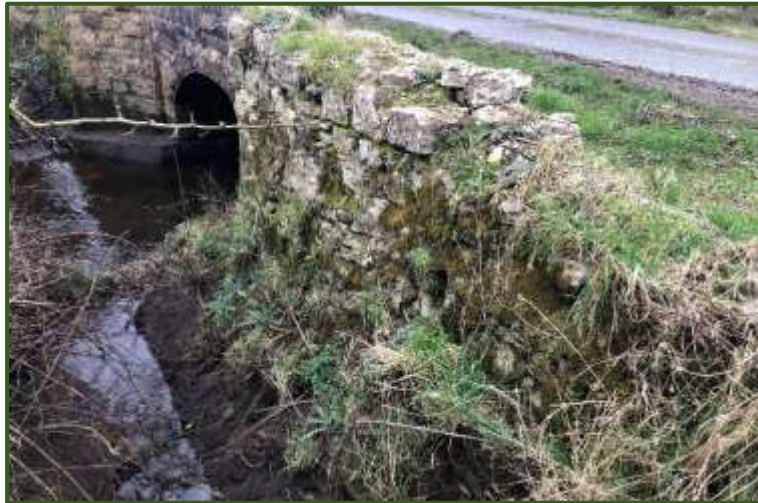
Picture 1: Image showing location of Lissanode Bridge prior to Bat Emergence Survey on 16/05/2024 the surveyor was positioned at this aspect
