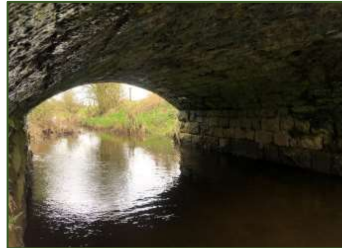
Picture 2: Image showing underpass of Lissanode Bridge; the image was taken from the north side of Lissanode Bridge
