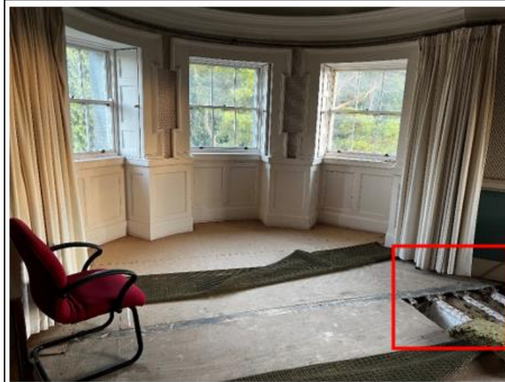
Plate 2 Evidence of bats accessing 1 st floor interior potentially through floor gaps/panelling.
