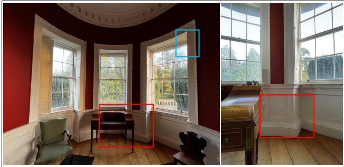
Plate 1 Ground floor – south-west bay area. Bats audible within the panel marked (red). Exterior roost entrance (blue).
