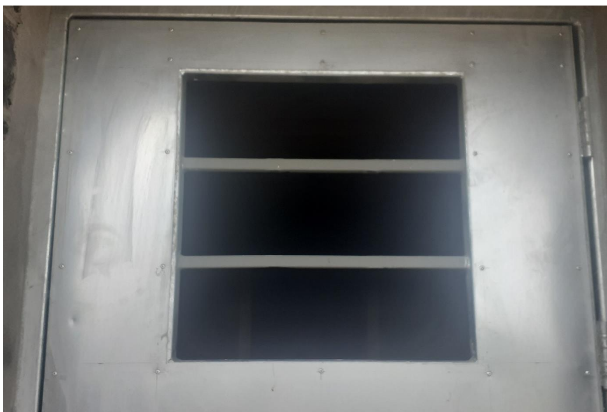
Plate 6: Example of post box entrance in door to allow bat movement between rooms.
