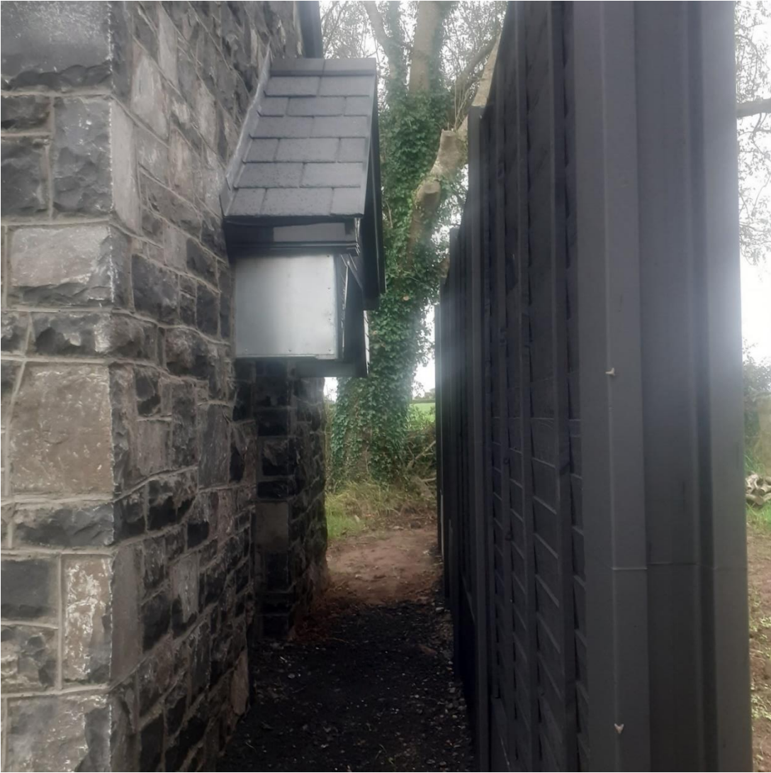
Plate 9: Partition wall constructed in front of entrance of Drim Bat House in County Clare – a similar structure is recommended around Griffins Cottage.
