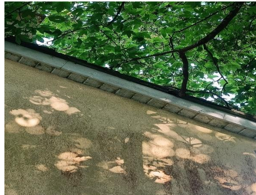
Plate 3-2 Gaps in the roof on western aspect of the dwelling.
