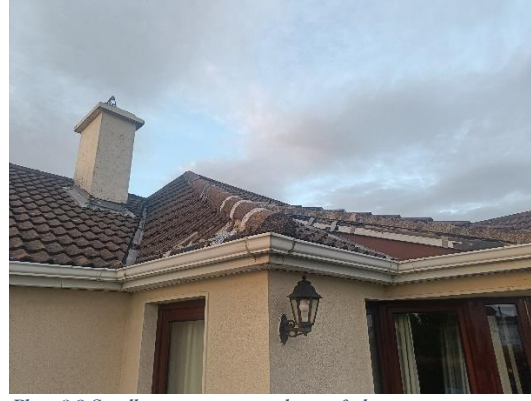
Plate 3-8 Small gaps present in the roof tiles.
