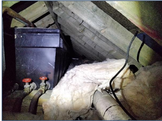
Plate 3 Three storey House: Attic space Section B and water tank – not accessed.
