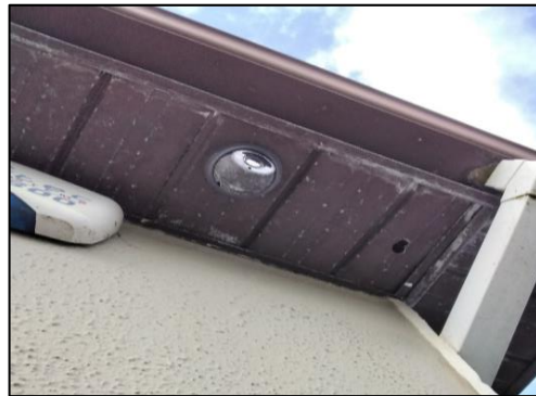
Plate 8 Southern aspect soffit with one hole.
