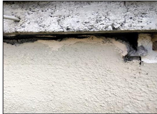
Plate 6 Three storey House: Small hole and crevice to the rear external wall.
