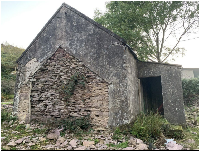
Plate 3-3: Gaps between stonework on gable end
