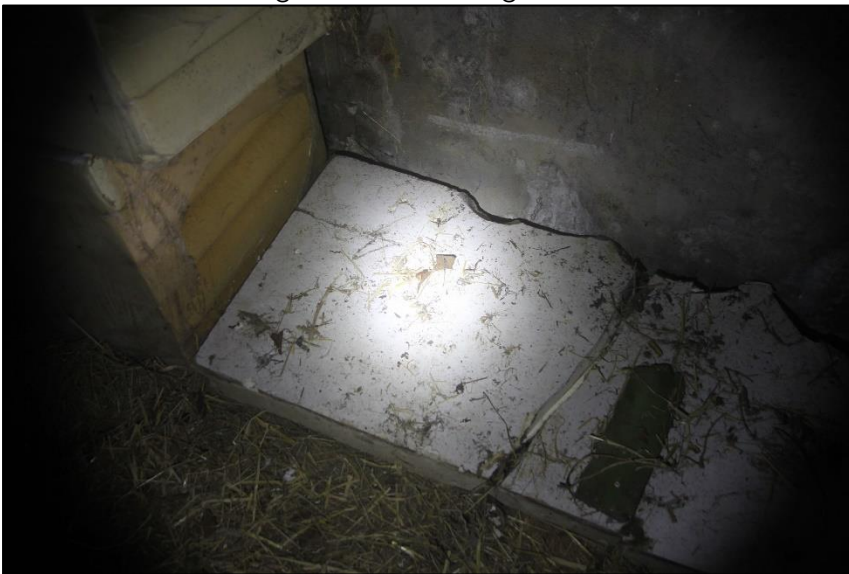
Plate 21 Building 1 Interior with bat droppings – August 2024
