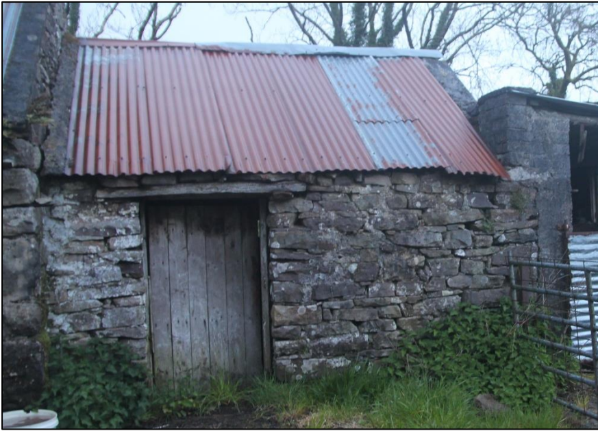
Plate 13 Building Labelled 3 – Moderate Roost Potential. Also used by nesting birds such as Barn Swallow. Access via back window when door is shut.
