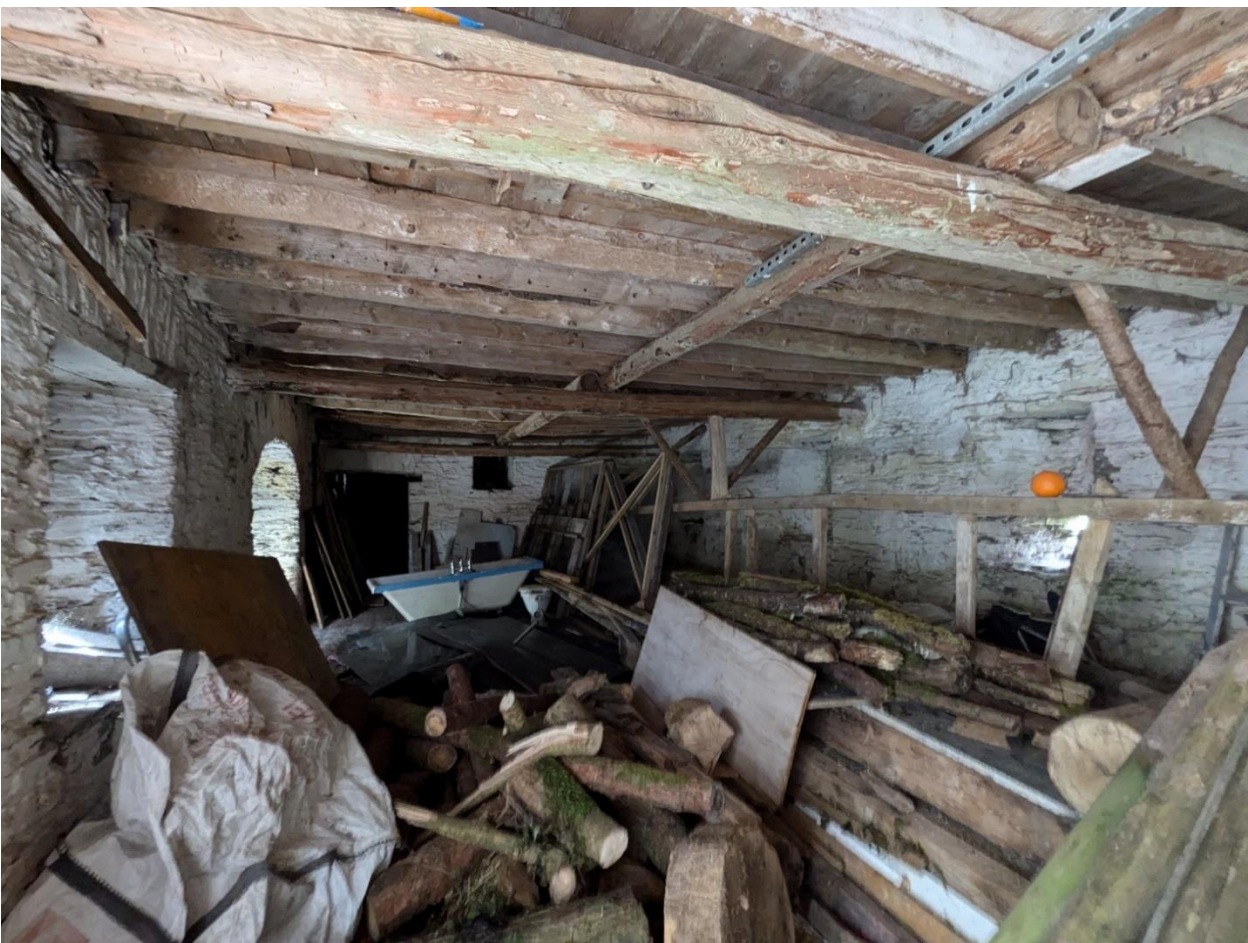
Figure 3-2: Cow byre building interior photograph of ground floor. A pool is proposed for this building.
