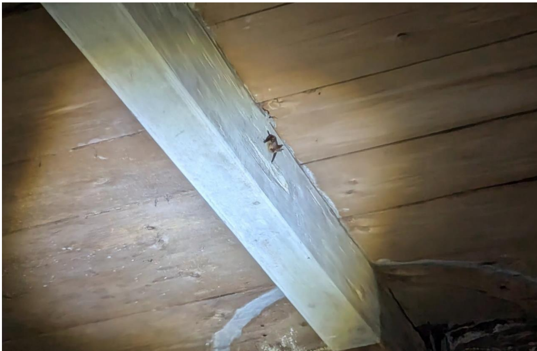
Figure 3-13: Brown Long-eared Bat recorded at 23:10 in the stables to be renovated for accommodation. This building is confirmed roost for BLEs.
