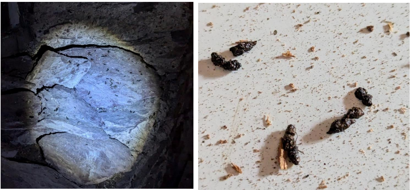
Figure 3-7: Bat droppings found in proposed 'Accommodation' building.
