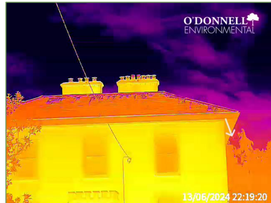
Plate 2.6 Thermal viewshed of camera overlooking the western aspect Lissardagh Main House, showing Whiskered Bat exiting from the southwestern portion of the fascia-soffit (white arrow).
