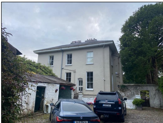
Plate 1 Eastern face of the subject house. During the activity survey a Soprano pipistrelle was often recorded foraging here.
