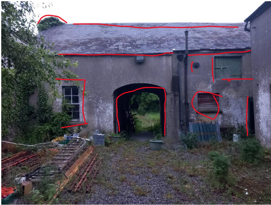
Figure 3-6 Rear facing garden – numerous crevices in stonework and in arch
