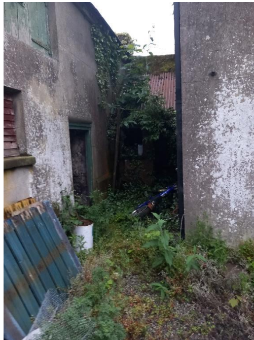
Figure 3-7 connecting shed proposed for demolition -low roost features due to light levels, damp and roofing material.
