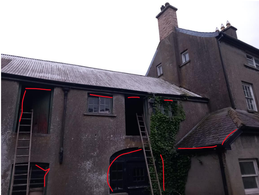
Figure 3-4 Building B1 (Outbuilding connecting to main house, proposed for renovation and extension, restaurant use) bat roost features
