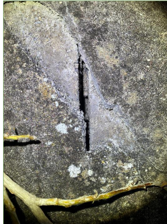
A8. A crack in the western gable of Hatchery 1 (see Plate 3.4 ) which gives access to cavity within the wall and was used by Soprano Pipistrelle for roosting on 31 st August 2022.
