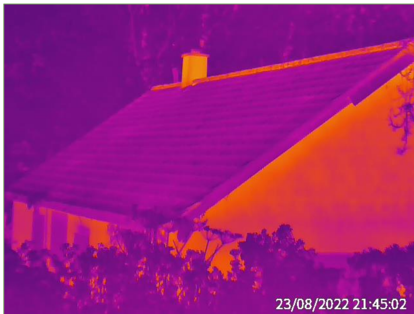
Plate 3.2 Example image from thermal camera placed on the north-eastern side of derelict residence.
