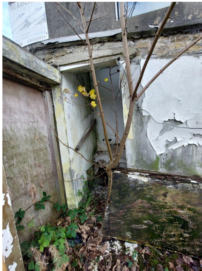
Photo 7: Stair access to first floor (steps rotten and collapsed)
