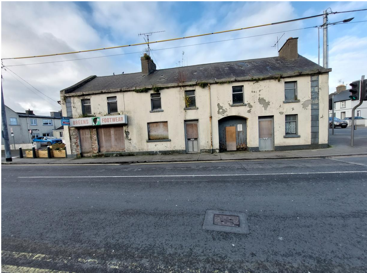
Photo 1: Front of building (adjacent to public footpath/road, roof structure sagging, roof tiles slipping. Gutters removed previously as they were collapsing onto public footpath below). The proposed new row of terrace houses will be narrower and offset further back from the public roadway.
