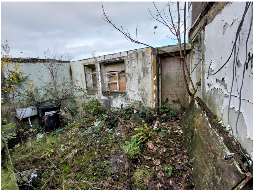
Photo 5: Rear room (roof structure collapsed, rubbish and vegetation collecting in area)
