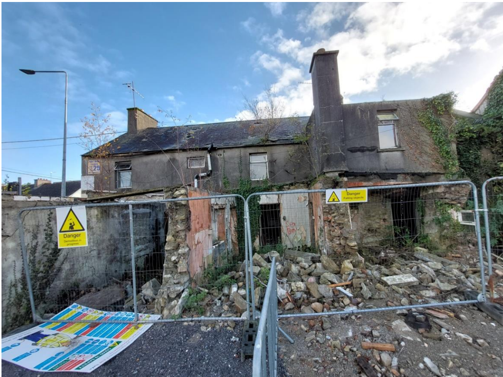
Photo 3: Rear Elevation of Buildings (roof collapsing, roof tiles slipping, access blocked to prevent falling objects, structure generally unstable throughout)
