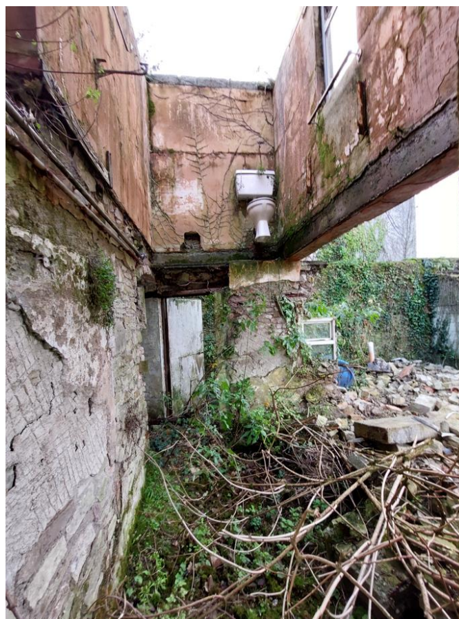
Photo 6: Rear room (roof structure and first floor structure previously collapsed, rear overhanging wall precarious and at high risk of collapse)
