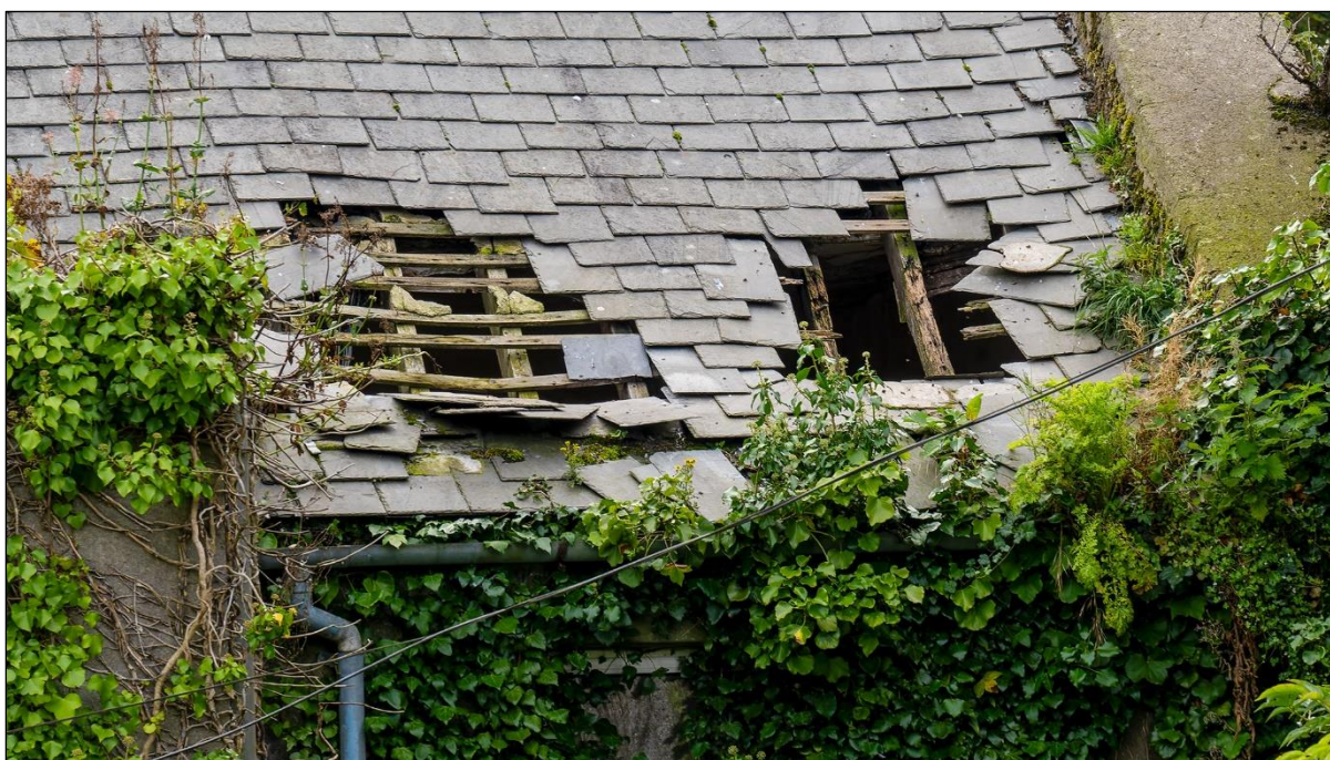
Plate 4 The subject building showing poor state of repair. The building was too dangerous to enter.
