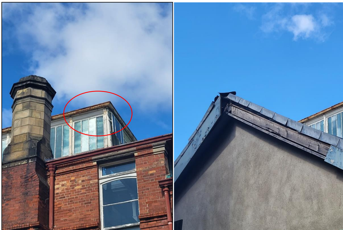
Plates 1&2 - The Anatomy Block (left) illustrating the location of a previously identified roost (red circle) on the northern end of the roof, and another section of the Anatomy building with loose flashing showing potential roost features (right)
