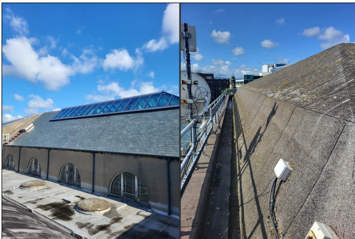
Plates 3 & 4. The roof of the former Medical Library Block, and a well-sealed section of the 1865 Block
