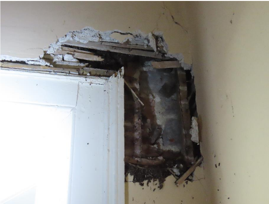
Photo 14 – bat droppings accumulated in space between wall and plaster
