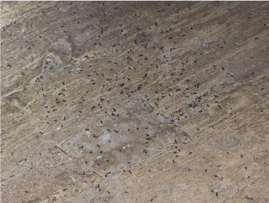
Photo 31 – bat droppings on floor of granary loft
