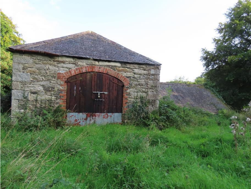
Photo 21 – rear elevation of main outbuilding. The granary loft is accessed via this door
