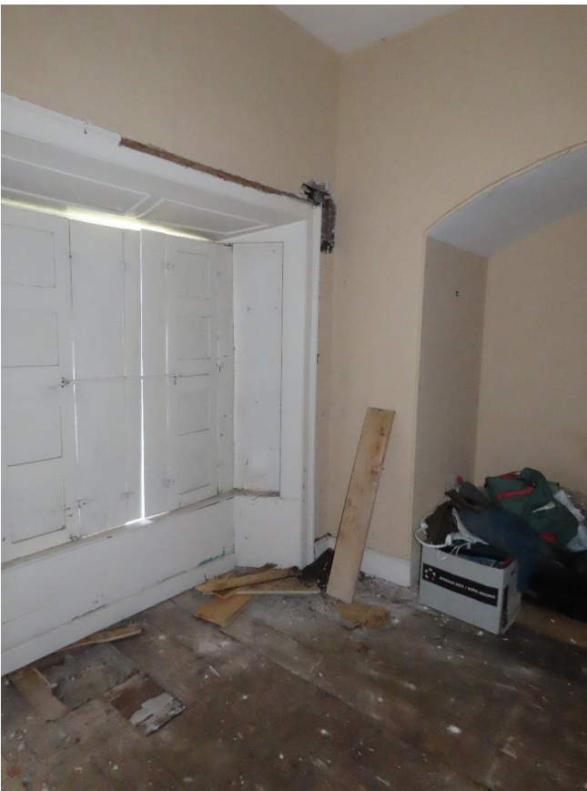
Photo 12 – section of plaster removed for architectural investigations in centre front bedroom. The pile of bat droppings are visible on the floor under the opening
