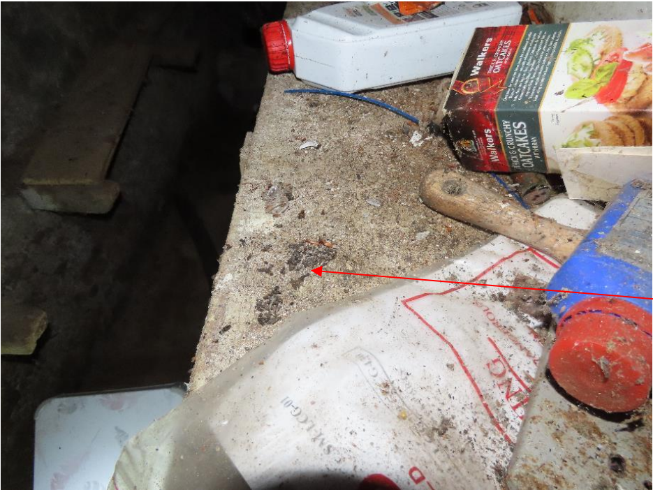
Photo 28 – bat droppings on work bench in workroom
