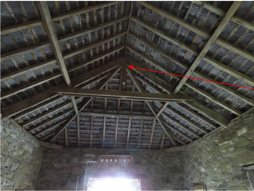
Photo 30 – hipped roof of granary. The position of the roosting Brown long-eared bats is indicated
