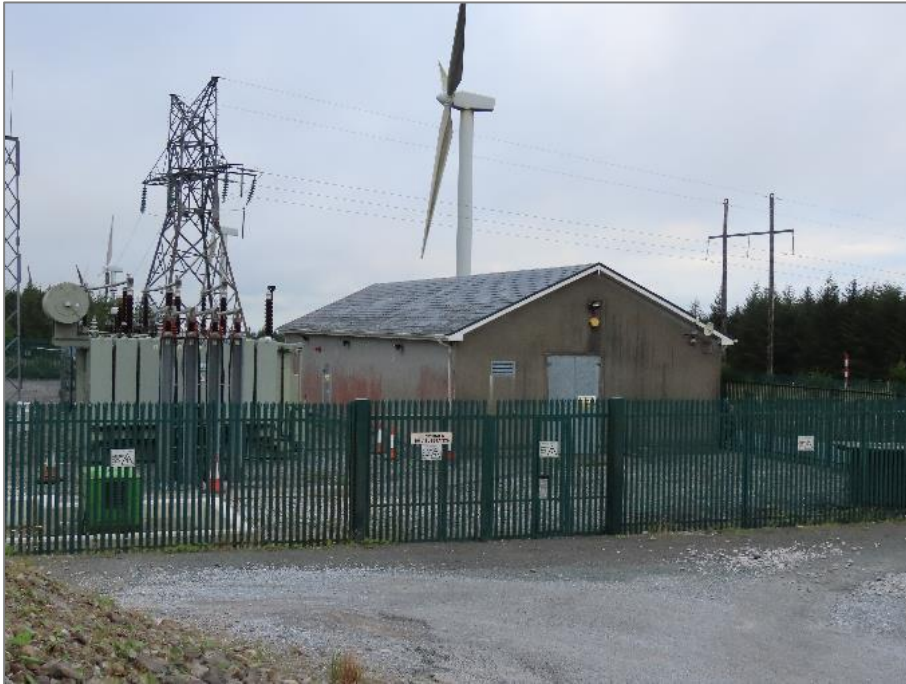
Photograph 1: Derrybrien Substation showing building and transformers (west elevation)
