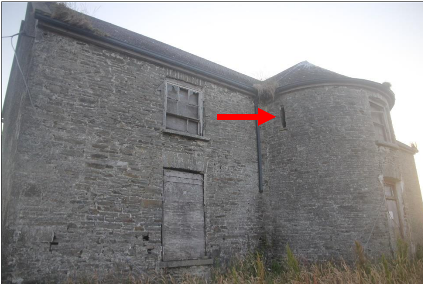
Plate 2 Side of front tower with access via both side window slits for bats and birds.
