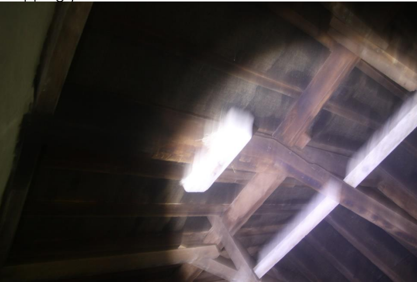
Plate 8 View from top of ladder into second storey of house with gaps evident between beams, potential roosting features.
