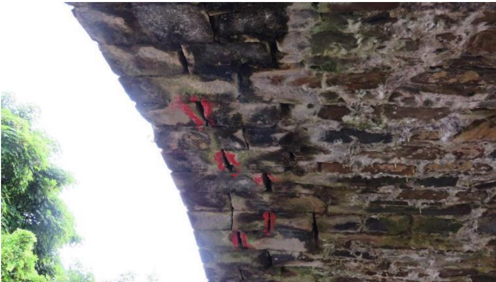
Five previously marked crevice behind the downstream facing stones of the western arch. A total of 17 Daubenton's bats were recorded in these crevices
