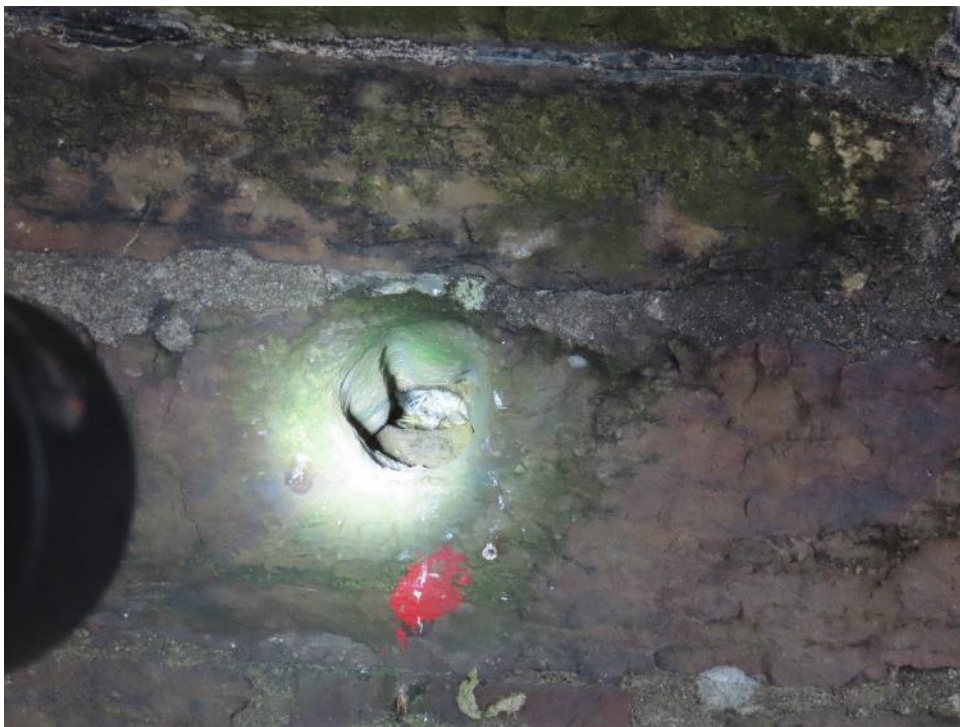
Duncannon Bridge – Sand martin nest in bore hole
