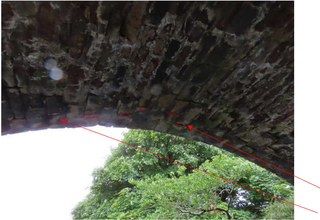
Duncannon Bridge – five crevices marked all behind downstream facing stones of westernmost arch
