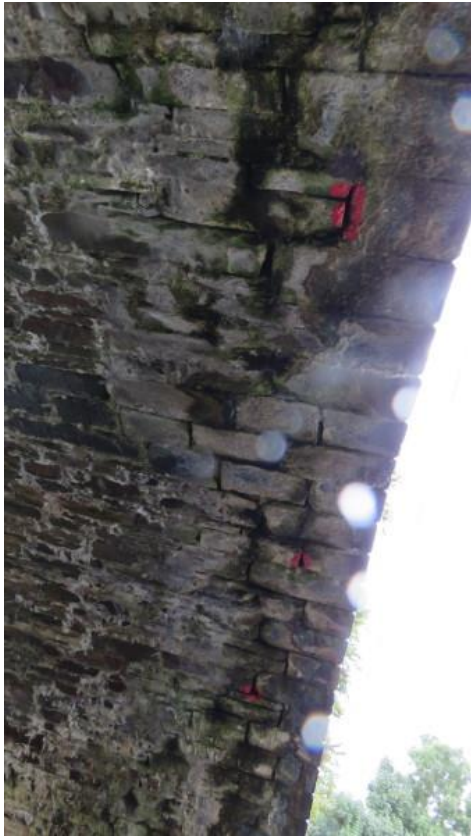
Photo 4 – Duncannon Bridge – 3 crevices marked behind facing stones
