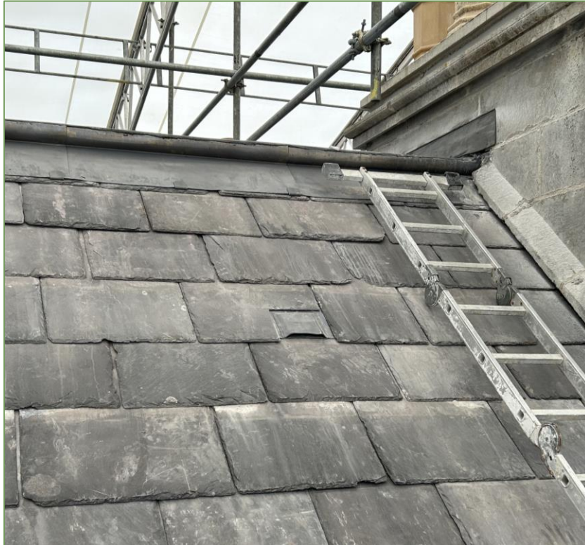
Plate 5.2 - Example of a lead bat access tile.
