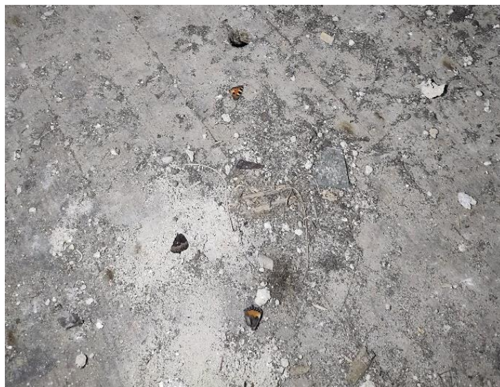
Figure 4: Insect wings and droppings on the first floor.
