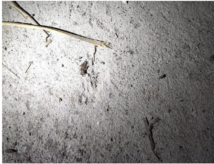
Figure 3: Bat droppings on the ground floor.
