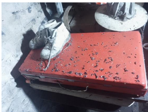
bat dropping in the shed which the loft opens out to (November 2024)
