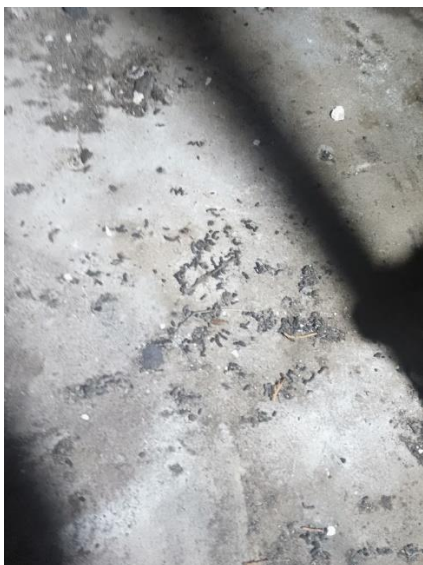
Bat droppings in the loft of the shed (November 2024)
